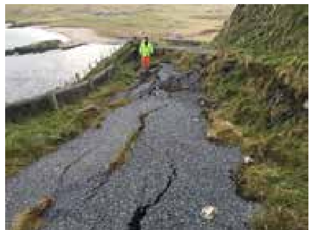
Photograph 32 Route option 6 – Section of damaged road
