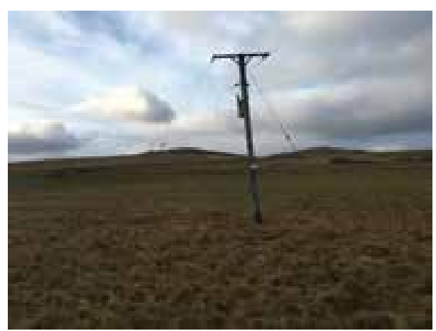
Photograph 06 – Overhead power line
