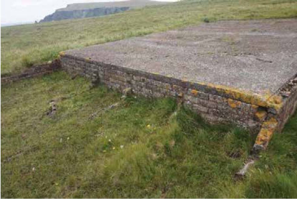
East face of west portion with failing joints and damaged brickwork.
