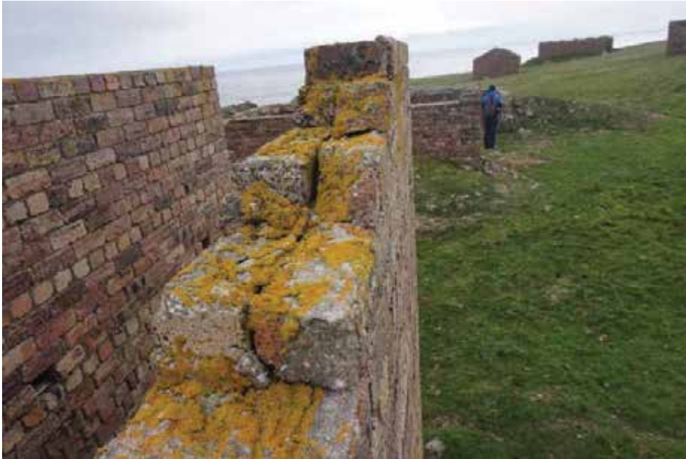
Failing skyward facing joints should be repointed.
