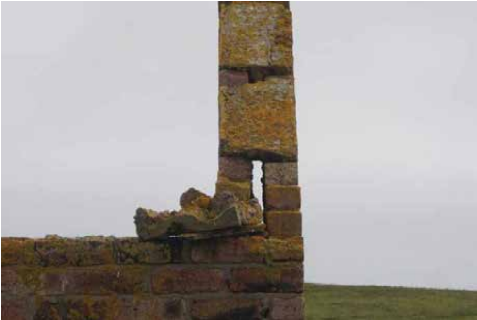
Damaged and dislodged concrete capping to south gable should be removed to reduce health and safety risk. Note that no wall ties are visible within the cavity. Reinstating the wallhead capping will prevent water ingress into the cavity.
