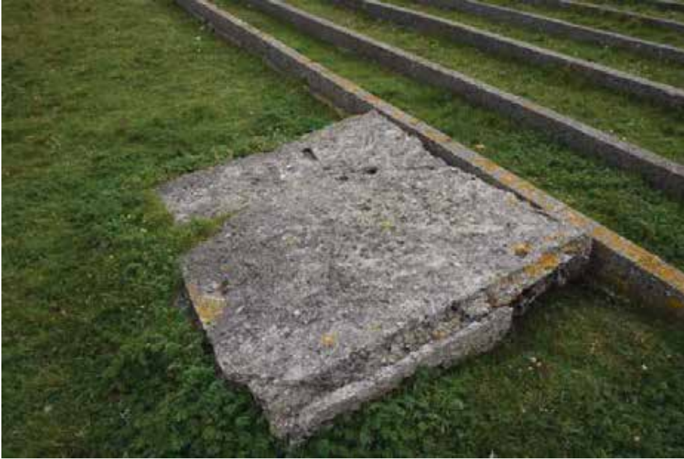
The entrance platt remains stable despite misalignment and localised cracking, spalling and disaggregation.
