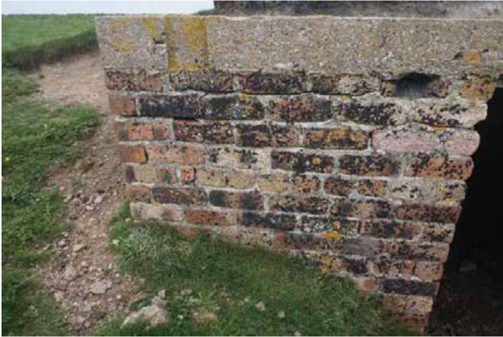
Cracked and failing mortar joints, and localised damaged brickwork.
