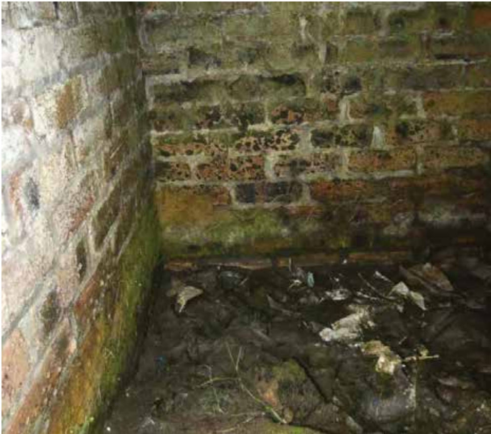
Saturated brickwork below covered area.
