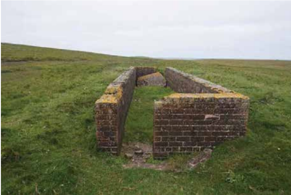
View from south showing missing wallhead brickwork, and displaced bricks and concrete roof slab.
