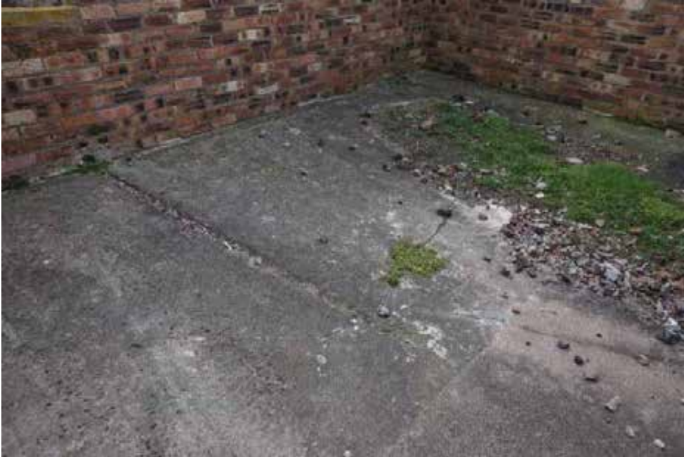
Cracked concrete floor slab supporting vegetation growth.
