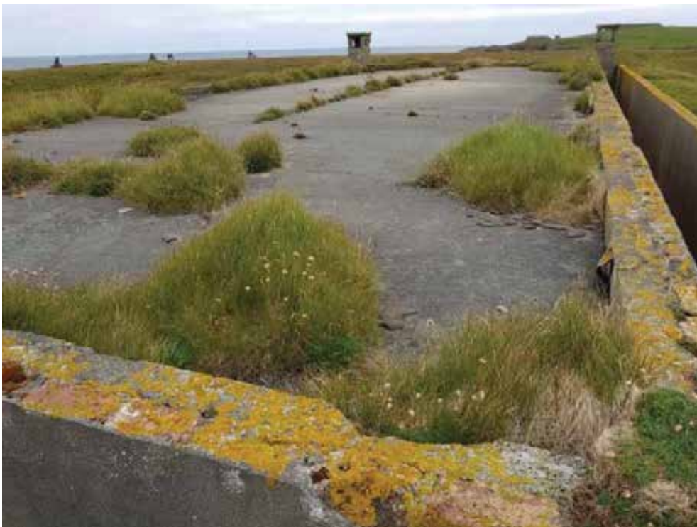
Looking across the roofscape. Note cracked asphalt, vegetation and missing concrete copes from wallheads.
