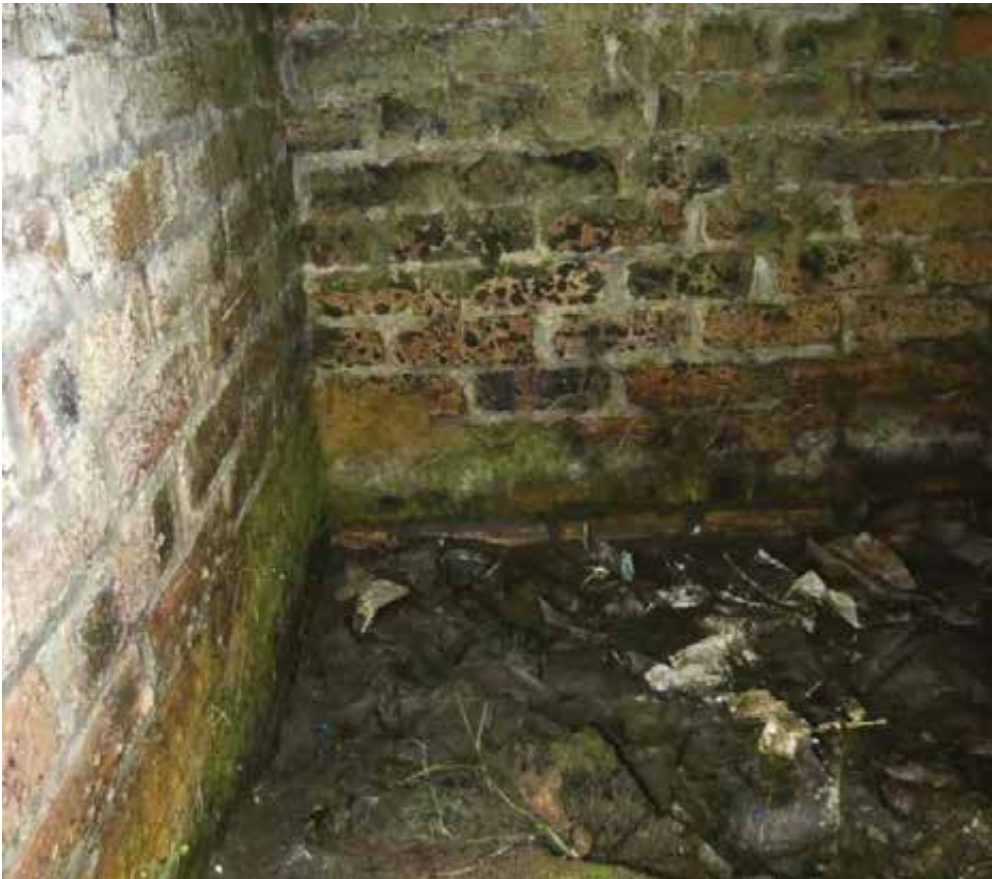
Saturated brickwork below covered area.
