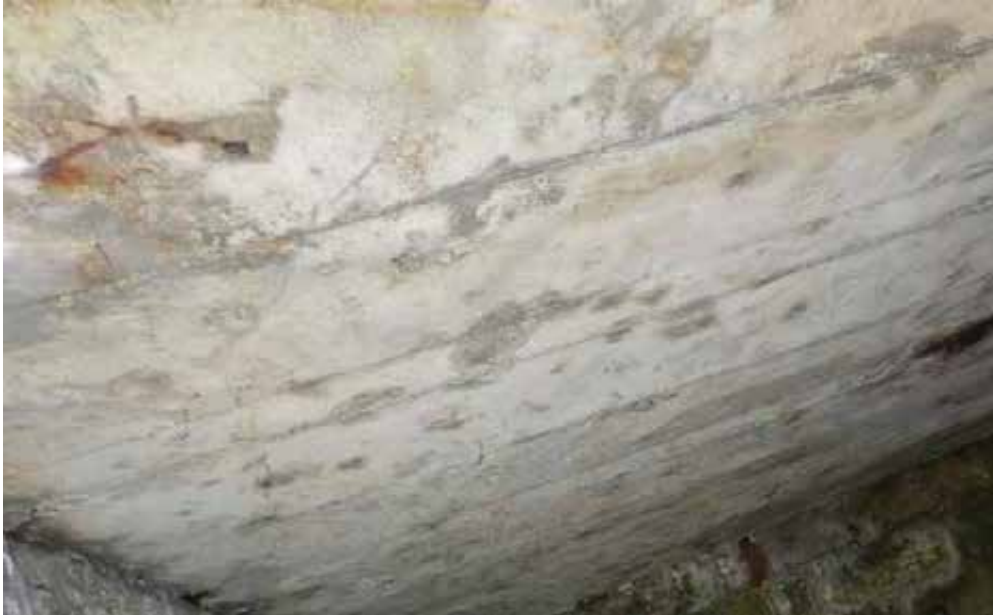
Minor spalling and exposed reinforcement.
