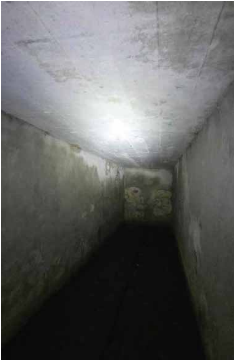
Localised failing render internally.
