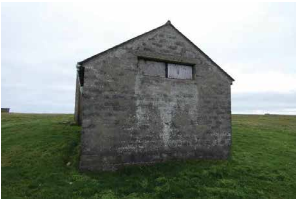
North elevation: Repoint cracked lintol and monitor. Replace boards to window and decorate.
