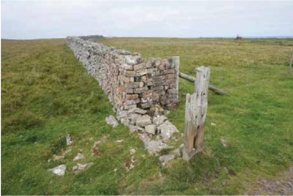
General view north: Brick repairs immediately north of the access road. The repairs remain functional. Rotten timber gate post.
