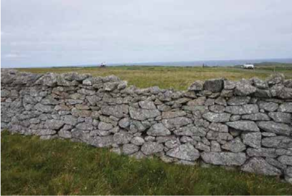
Displaced cope stones should be reinstated.
