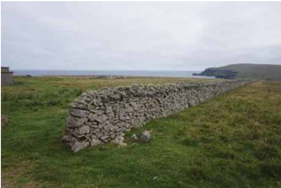
General view south: Copes should be regularly check and loose/displaced stones reset.
