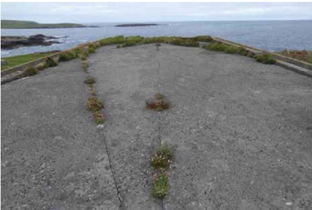
General view across the roof. Note cracking of the asphalt and vegetation growing from those cracks.
