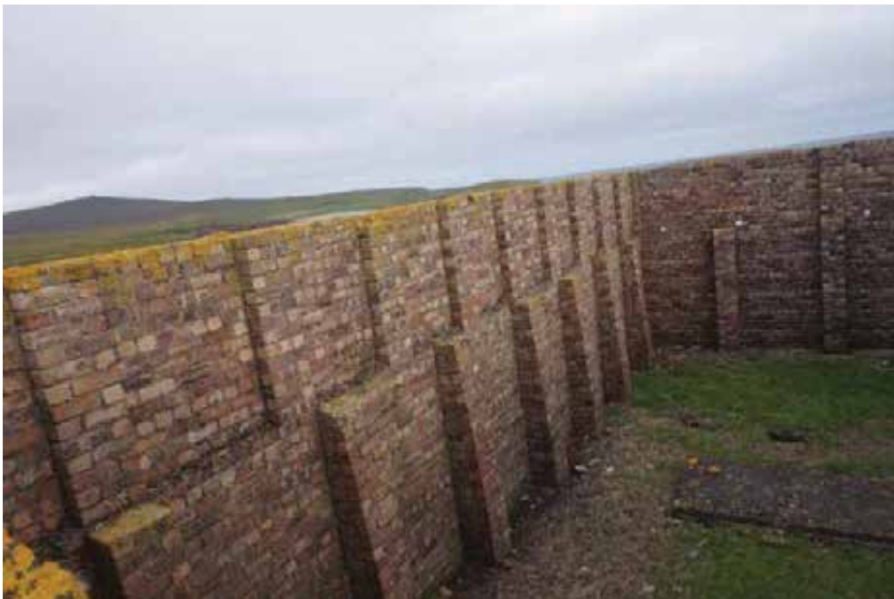
Cracks at higher levels are aligned with the upper piers which are poorly tied to the adjacent thinner single brick thick infilled brickwork. See also Photo 2
