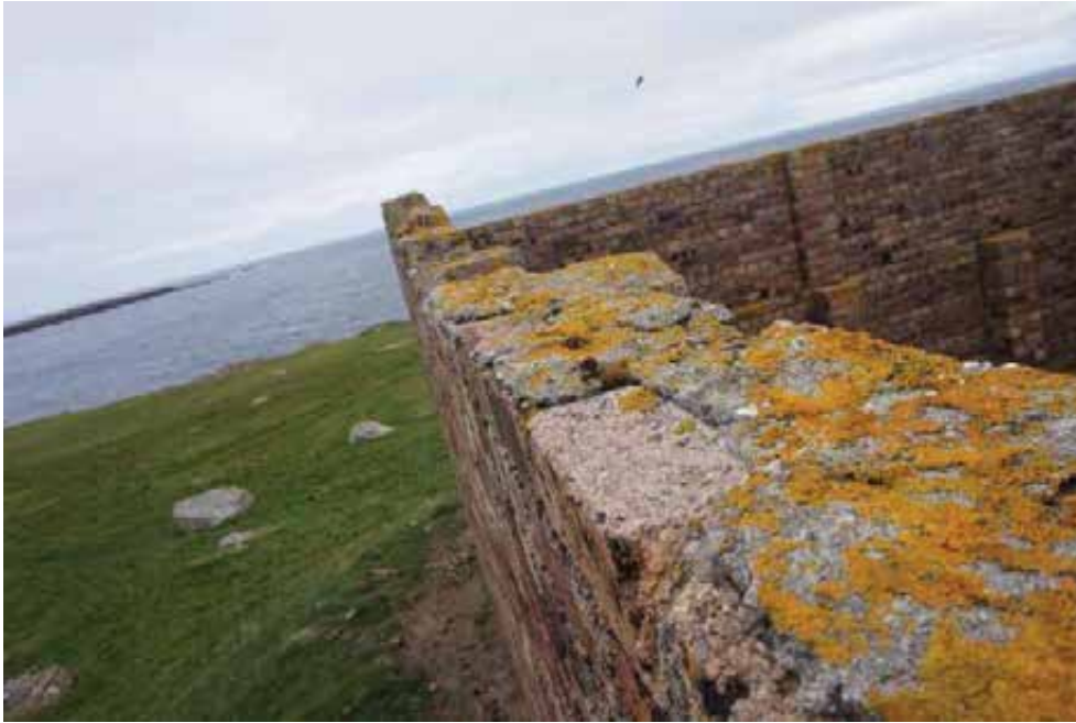
Failing skyward facing joints should be repointed, with allowance for rebedding loose bricks.
