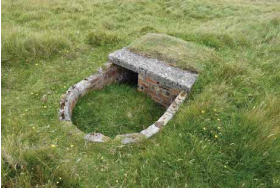
General view. Note damaged wallhead bricks.
