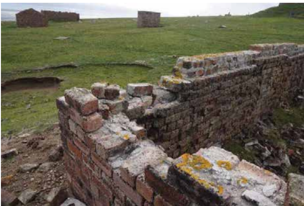
Loose wallhead brickwork and failing joints.
