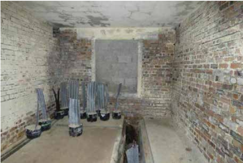
As 10. Note cracked ceiling plaster and indications of general dampness in the brick masonry.
