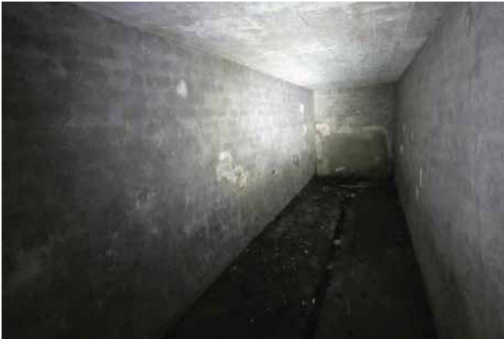
Localised failing render internally.
