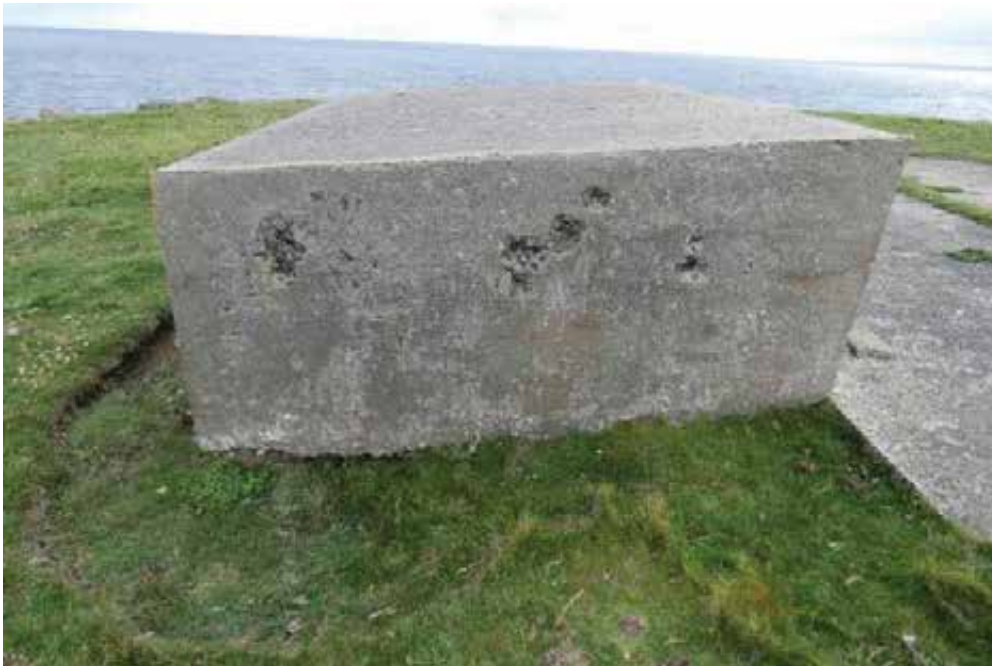
Localised spalling and damage to external walls.
