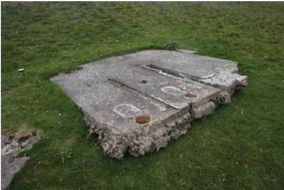
East concrete base with spalling upper face.
