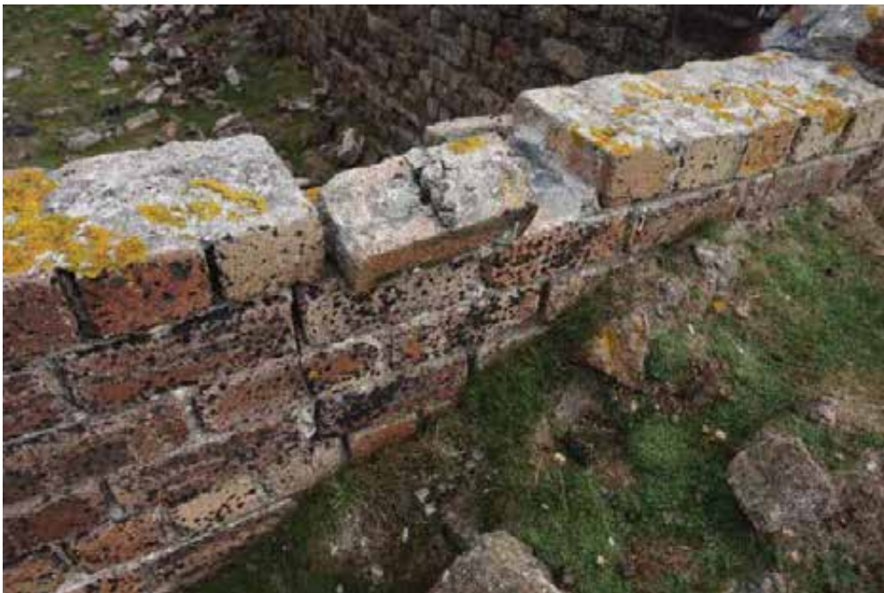
Defective skyward facing joints should be repointed, with allowance for resetting loose brickwork.
