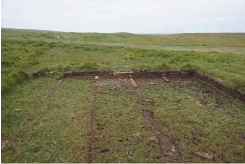
Internal view showing part buried footings with loose bricks and failing mortar joints. Note displaced brickwork. Consideration should be given to burying them to protect them from exposure to weathering and from the impact of increased footfall to the site.
