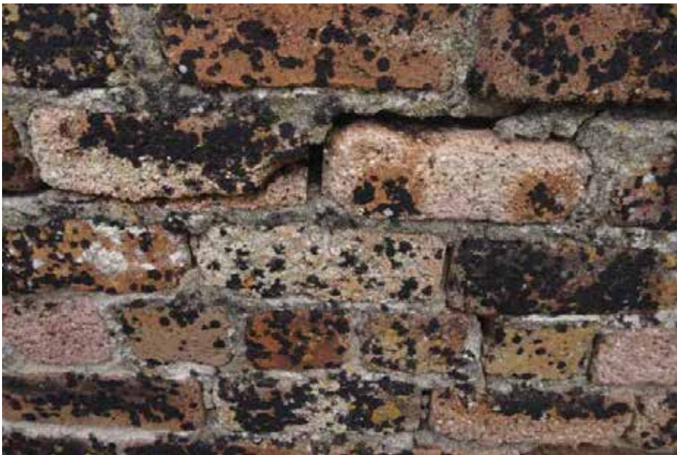
Damaged areas should be repointed to minimise further damage from water ingress and freeze/thaw.
