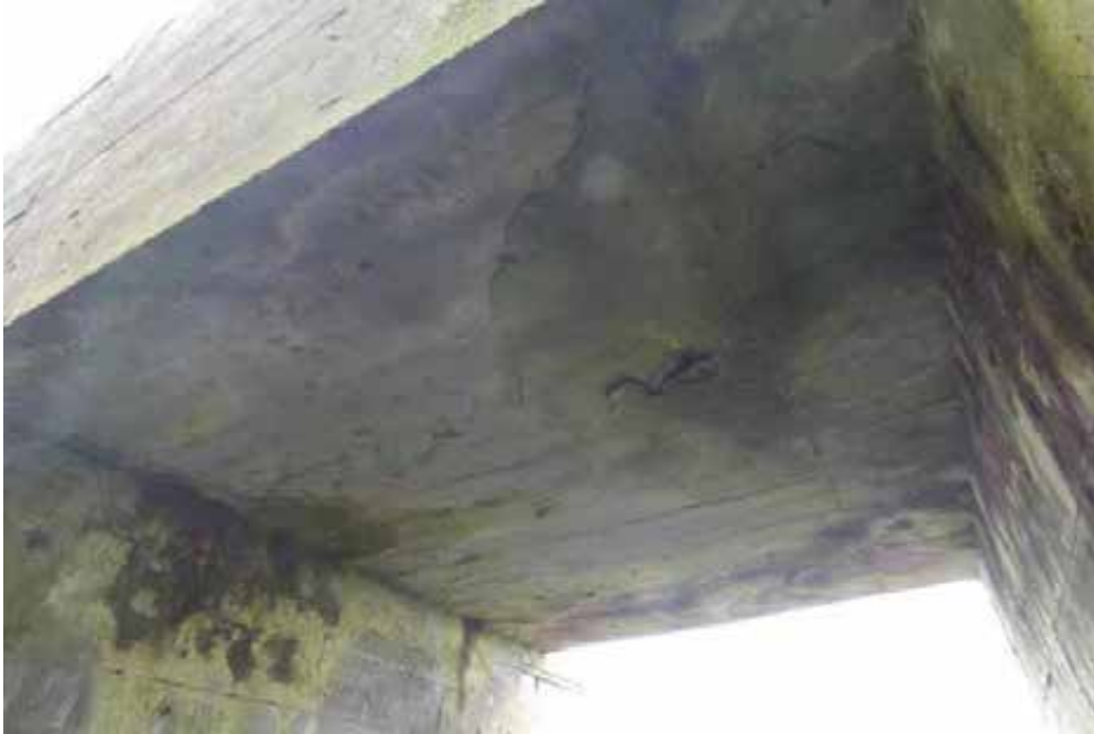
Spalling concrete and render finishes from the soffit of an access tunnel roof.
