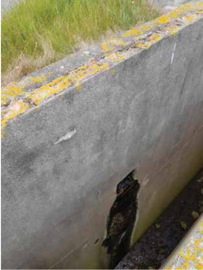
The outlet from the roof runs down into the wall and discharges part-way up it. Outlet is blocked by vegetation. Not loss of render from below the discharge point.
