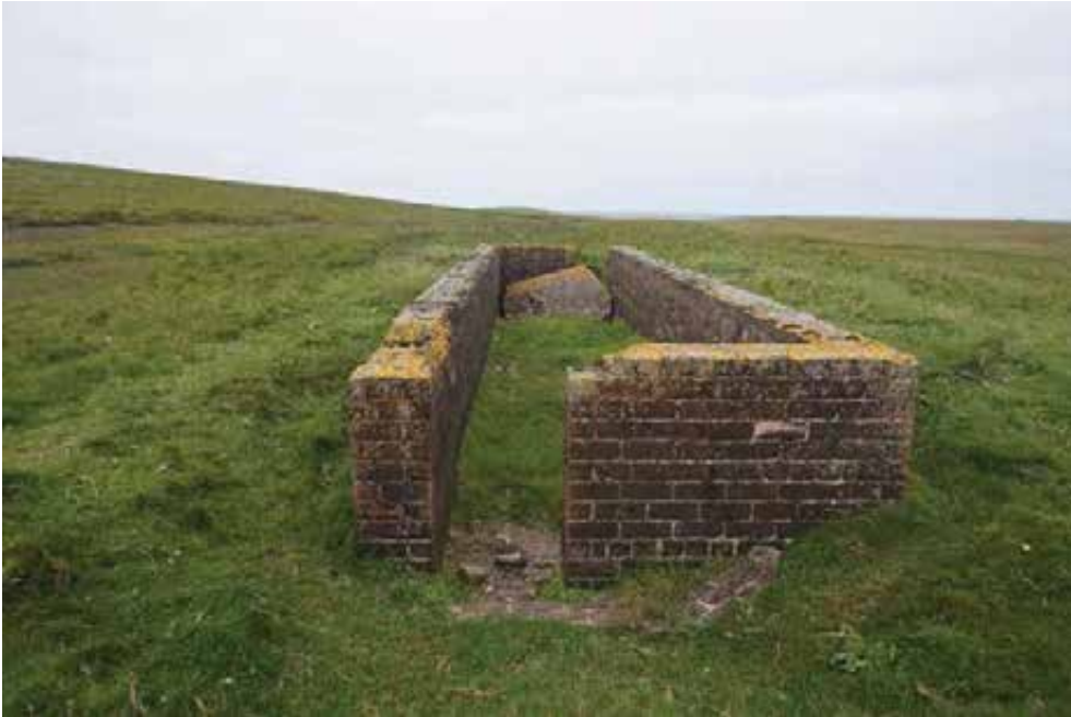
View from south showing missing wallhead brickwork, and displaced bricks and concrete roof slab.
