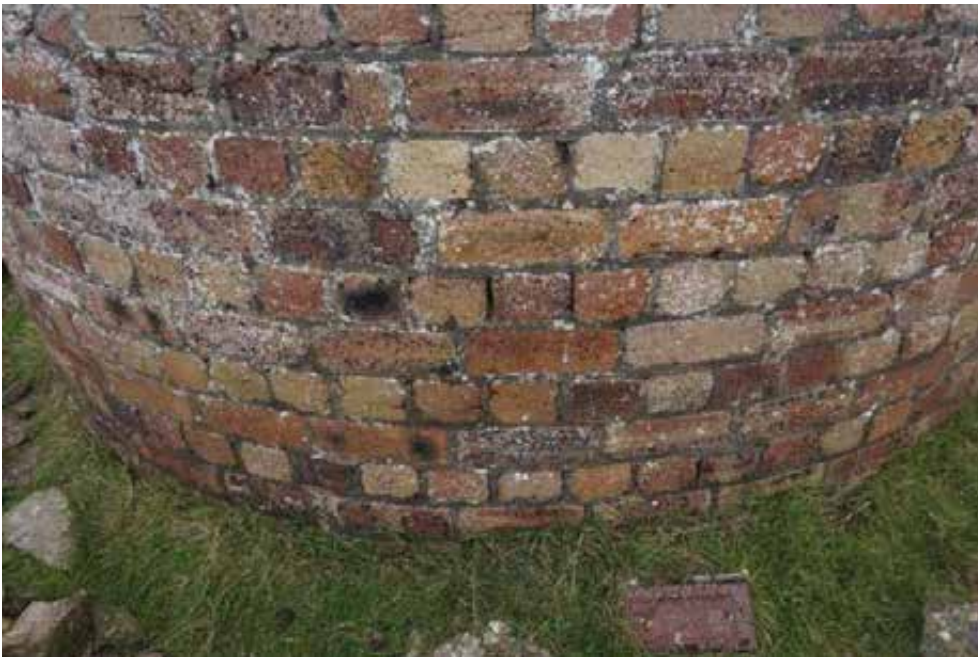
Localised failing joints to wall face.
