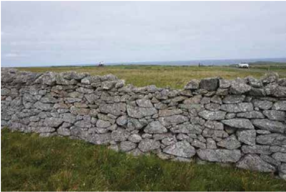
Displaced cope stones should be reinstated.
