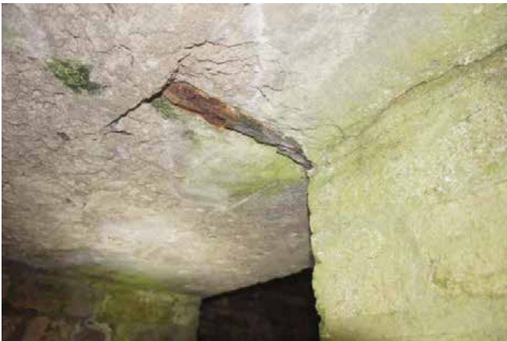
Despite the lack of roof finishes, only minor corrosion of reinforcement was observed.
