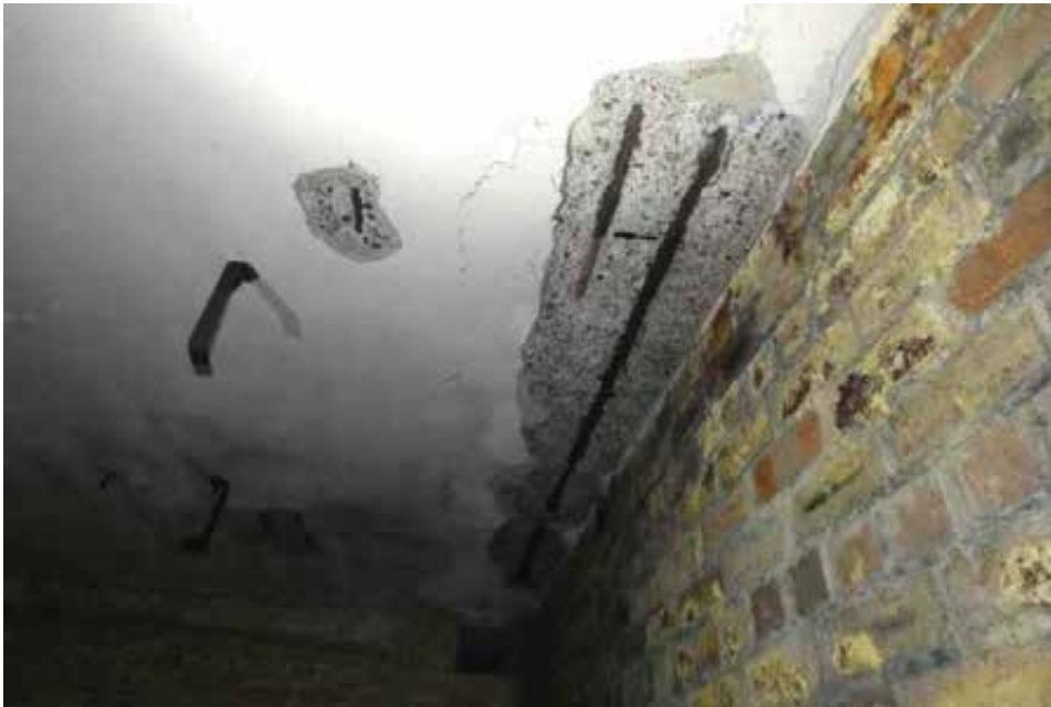
In places, expansive corrosion of reinforcement is causing spalling of concrete from roof soffit.
