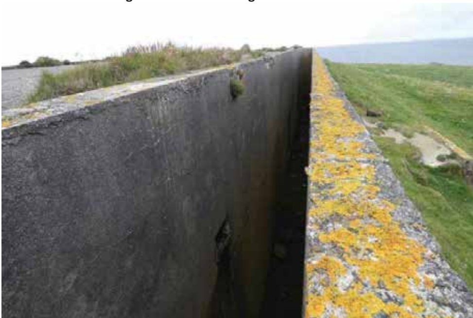
From the top of the embankment looking down into the gap between blast wall and building. The discharge point from the rainwater roof outlet can be seen partway down the wall of the building. Vegetation growing from this outlet is blocking it.
