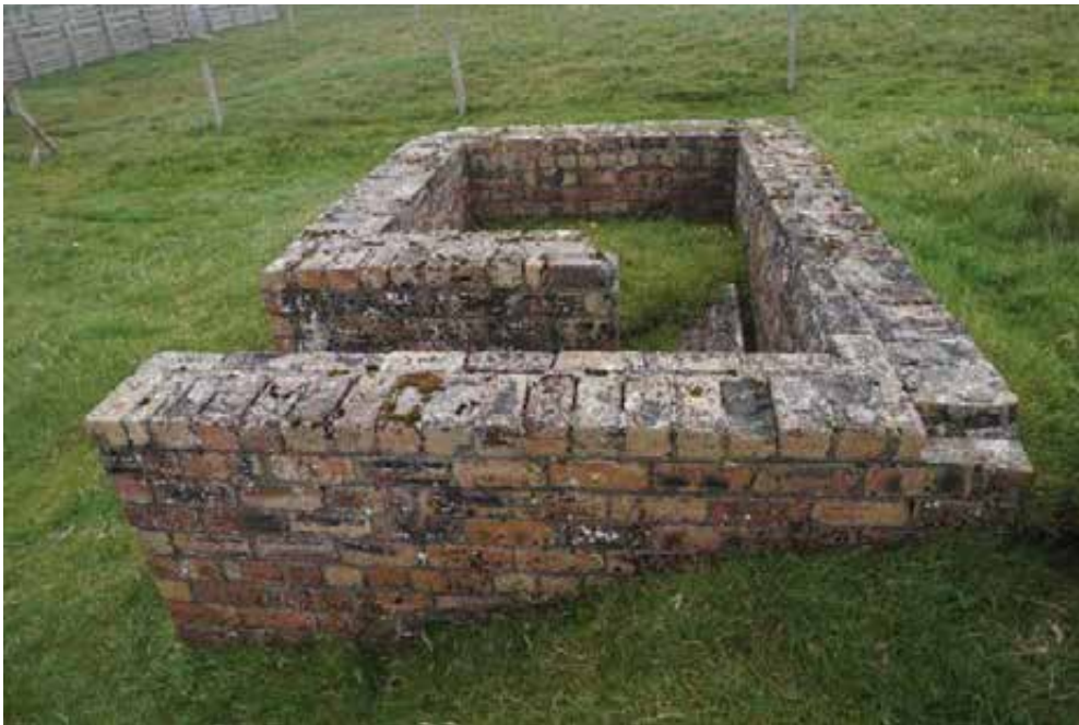
North Elevation: Missing and damaged brickwork and defective mortar joints.
