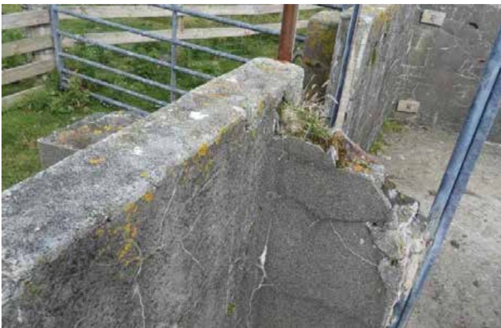
Localised damaged wallhead brickwork.
