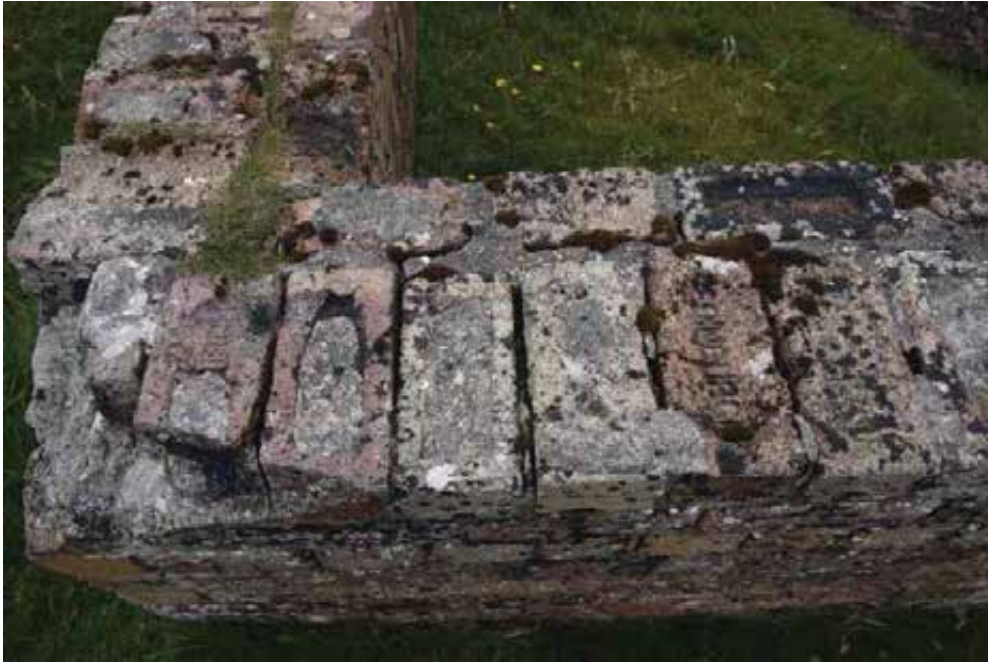
Open and defective wallhead joints and damaged brickwork in southeast corner.
