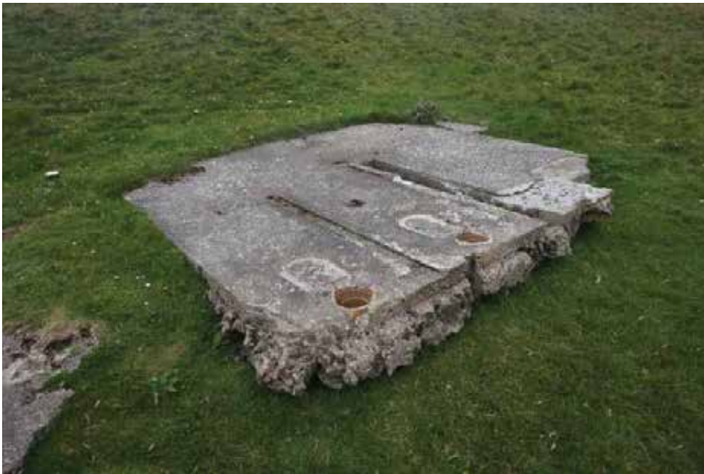
East concrete base with spalling upper face.
