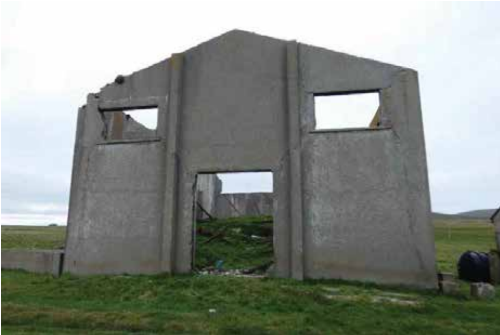
East elevation. Note the vertical cracking at each corner. Note the diagonal cracking between the entrance opening and both window openings and how this cracking continues up to wallhead: this elevation is a stack of independent, thin, tall, wall panels sitting atop each other.
