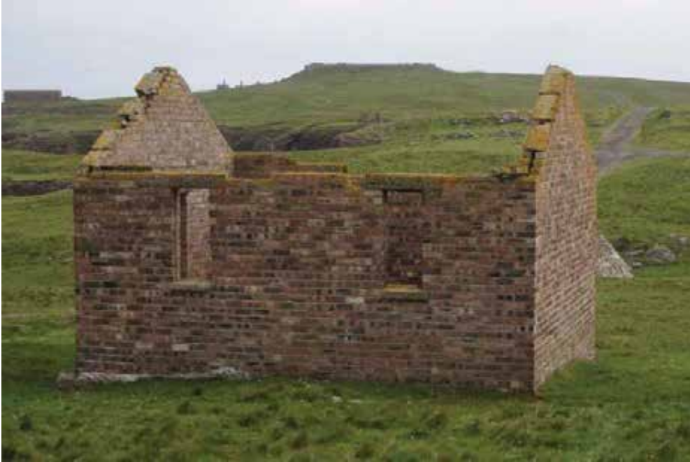
West elevation with missing wallhead brickwork. Note failing cappings to gables.
