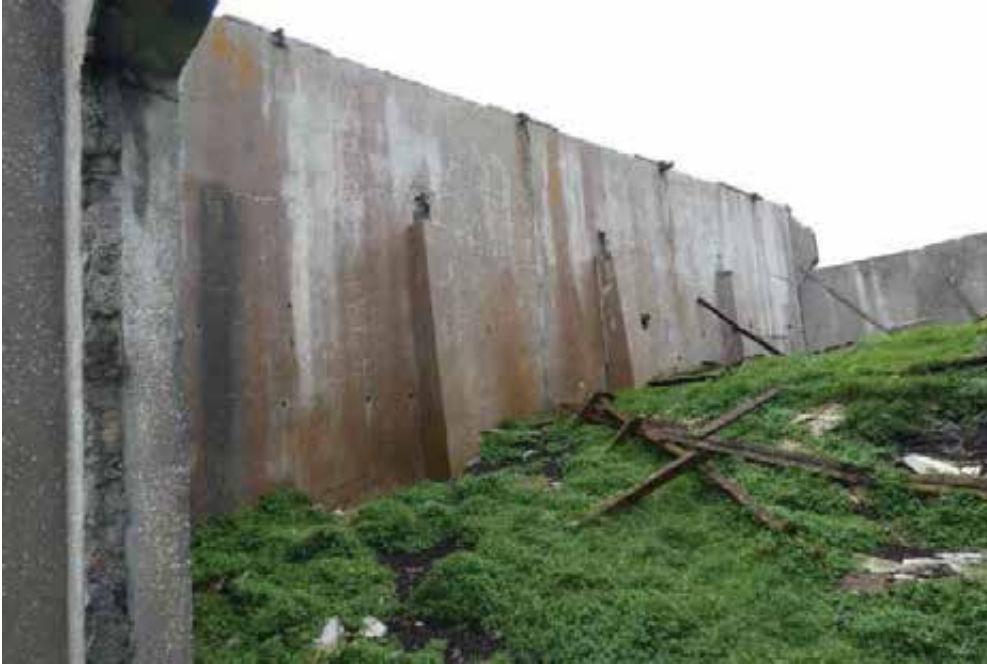
The internal piers do not appear to be fully or properly bonded to the masonry of the external walls.
