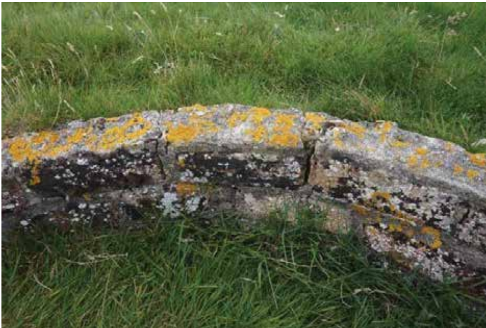
Localised failing joints to wallhead of curved west end.
