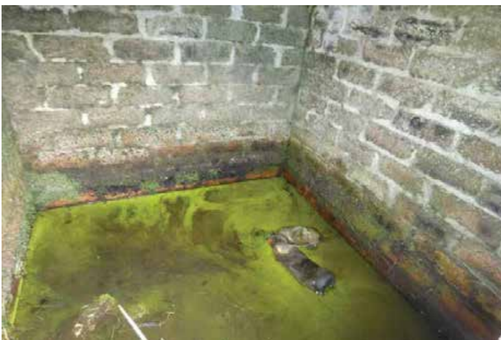
Flooded covered area saturating brickwork above.
