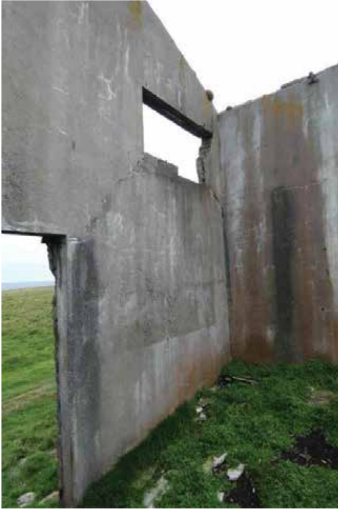
Internal view of east gable. Note how the cracking is right through the masonry.
