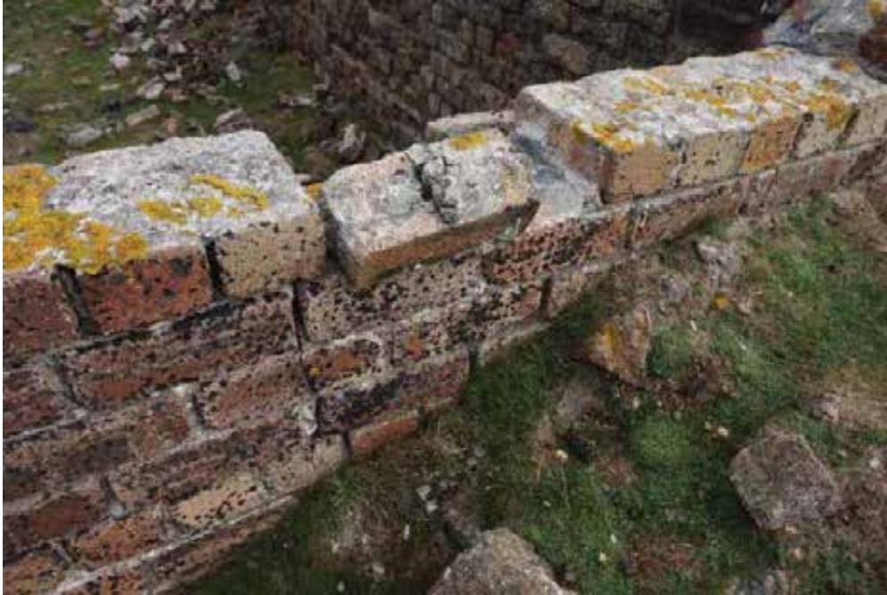
Defective skyward facing joints should be repointed, with allowance for resetting loose brickwork.
