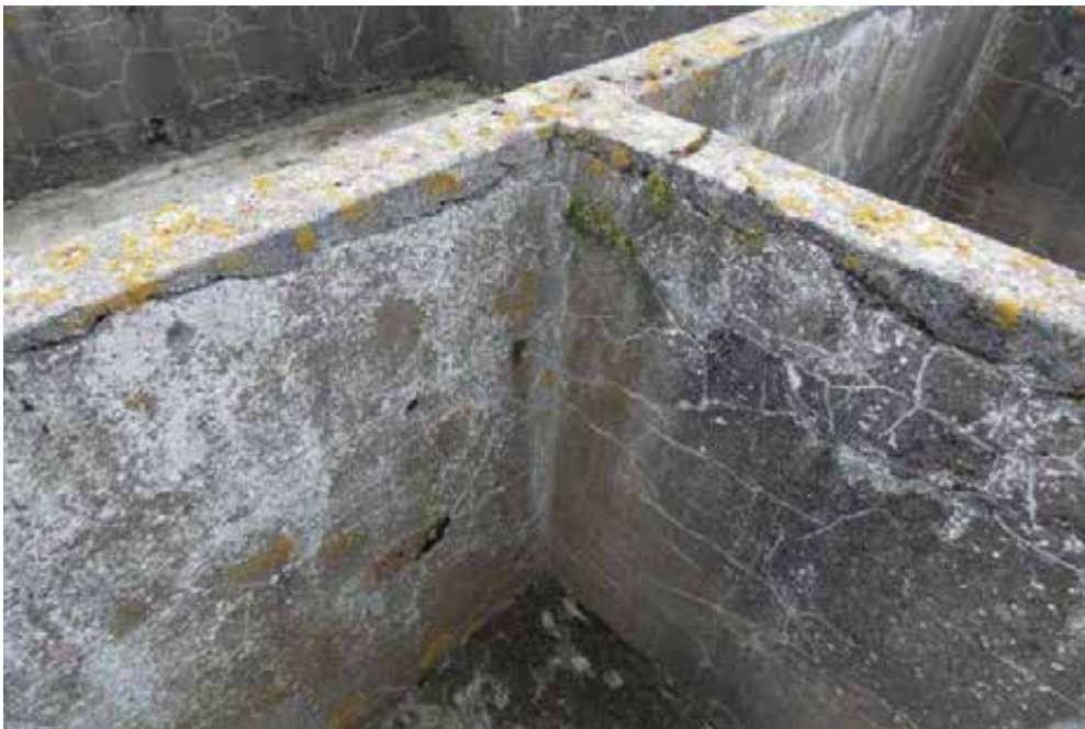
The render was patch repaired when the walls were lowered. All render (original and later) has cracked.
