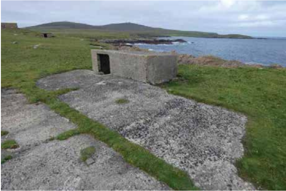
General view showing cracked hardstanding which is supporting vegetation growth.
