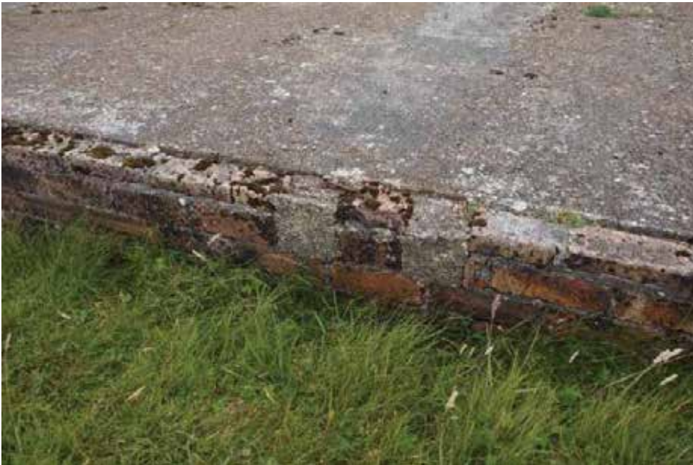
Stumps of reinforced concrete superstructure visible on the footings of the north and south elevations. Note cracked and failing mortar joints.
