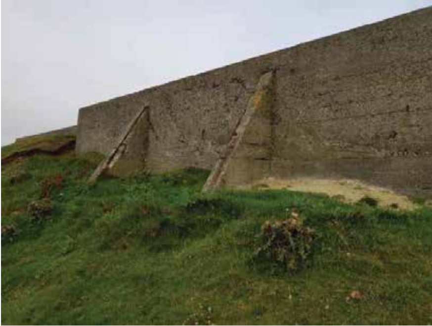
RC buttresses to the blast walls of the south side of the structure.
