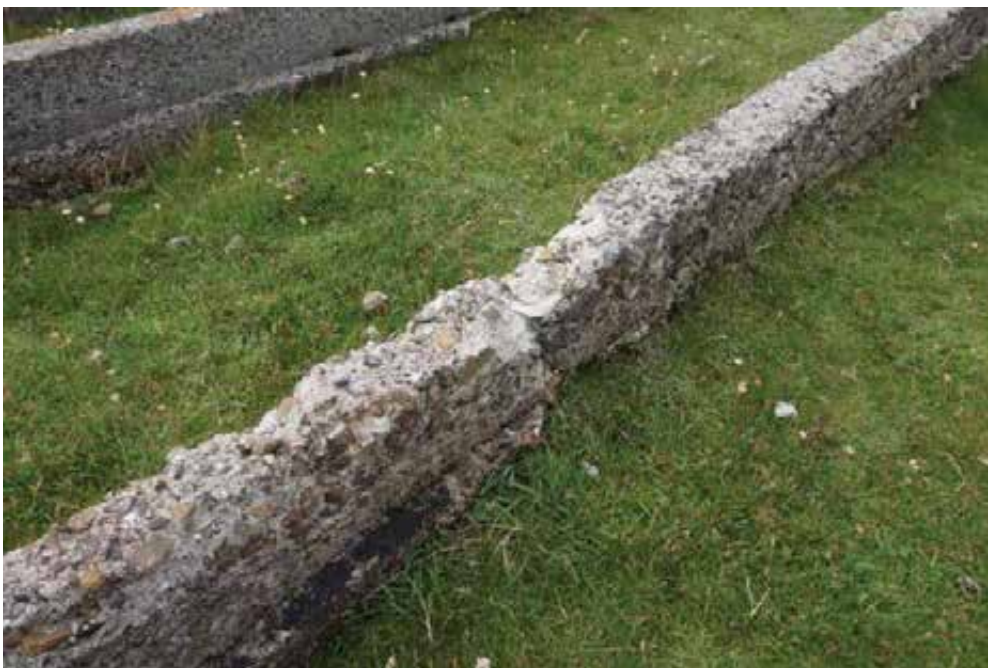
Localised spalling and disintegration at the eastern end of one of the centre sleeper walls.
