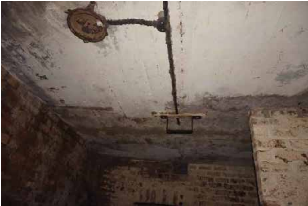
Corroded surface mounted servicing.
