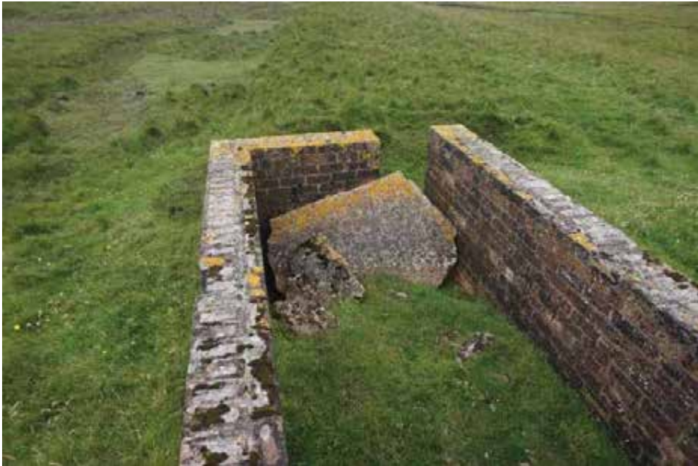
Internal ground levels have increased due to accumulations of soil, and fallen brickwork and concrete.
