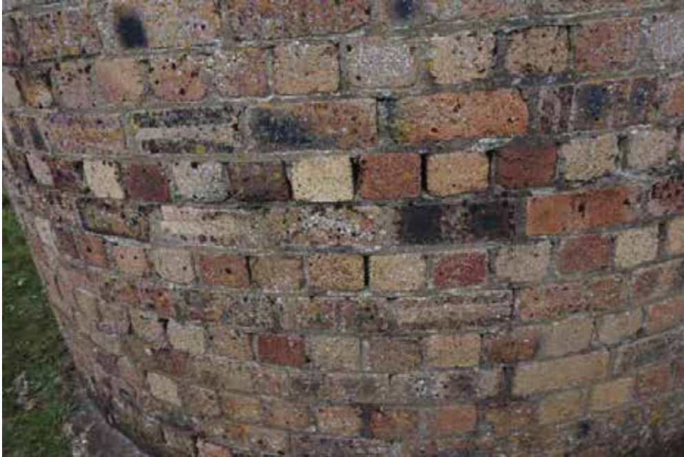
Localised failing wallface joints.
