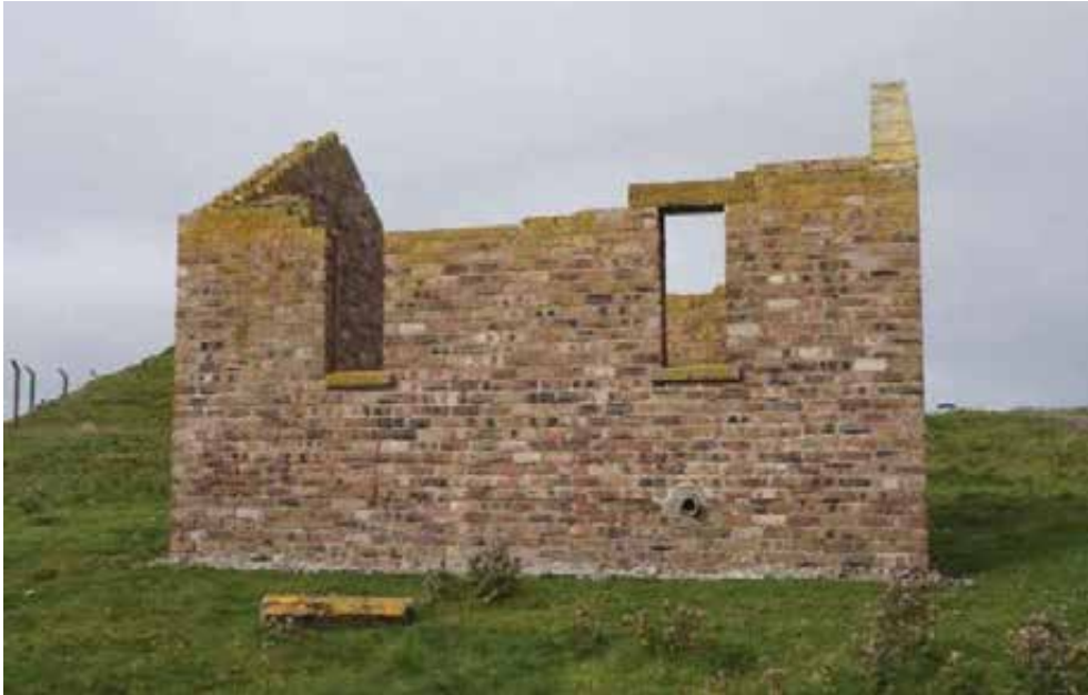
East elevation with dislodged lintol and fallen wallhead brickwork. To prevent ingress into the cavity, consider resetting the lintol and brickwork to allow the wallhead to be capped in concrete.
