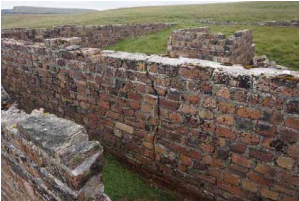
Cracked brickwork to the single brick thick east facing inner skin. Cracks should be repointed to allow future monitoring.
