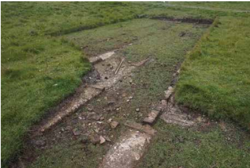
Loose brick footings, disaggregated concrete strip foundations and displaced bricks, timber and metal work at southern portion of the structure.
