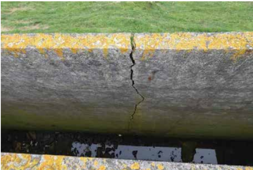
Vertical cracks in the blast walls are wider at the top of the wall than the bottom, indicating foundation movement. the provision of horizontal reinforcing bars appeared to be small.
