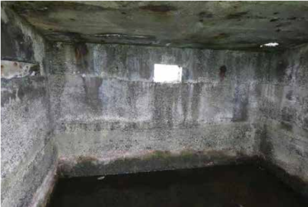
Hairline cracking, rust staining, leaching and discolouration to the walls exacerbated by flooding internally.
