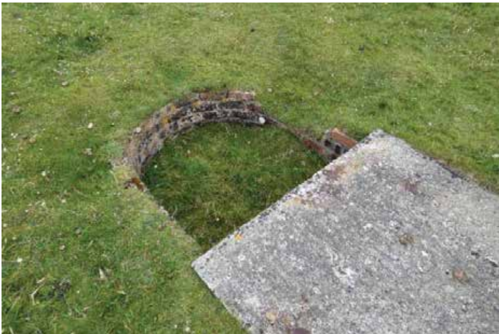
Missing wallhead brick work and defective mortar joints. Localised rust staining to concrete roof slab.
