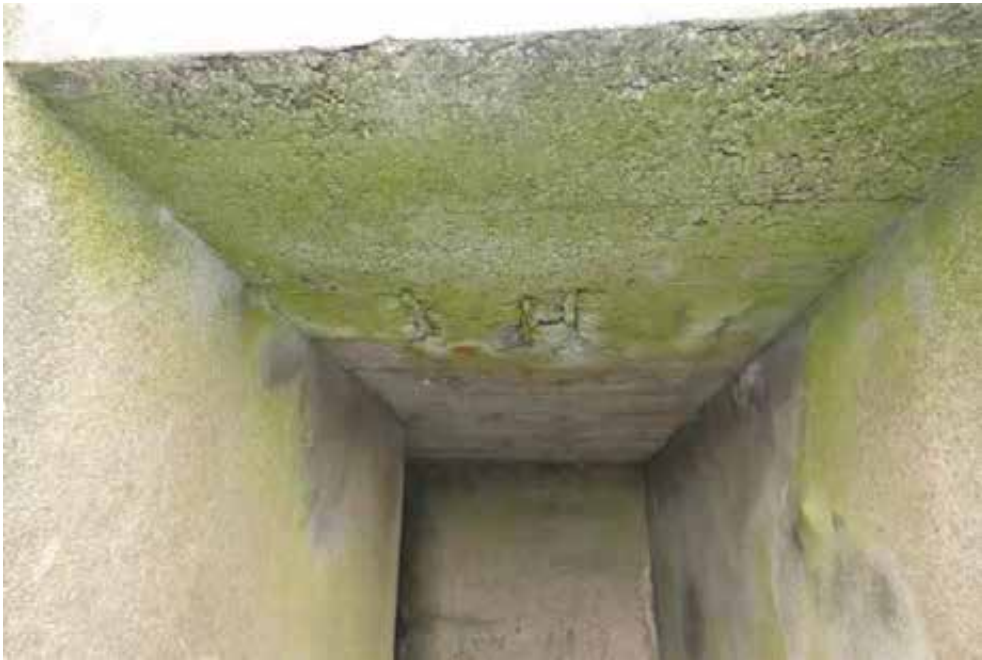
Localised spalling to the soffit of the roof slab exposing reinforcement.
