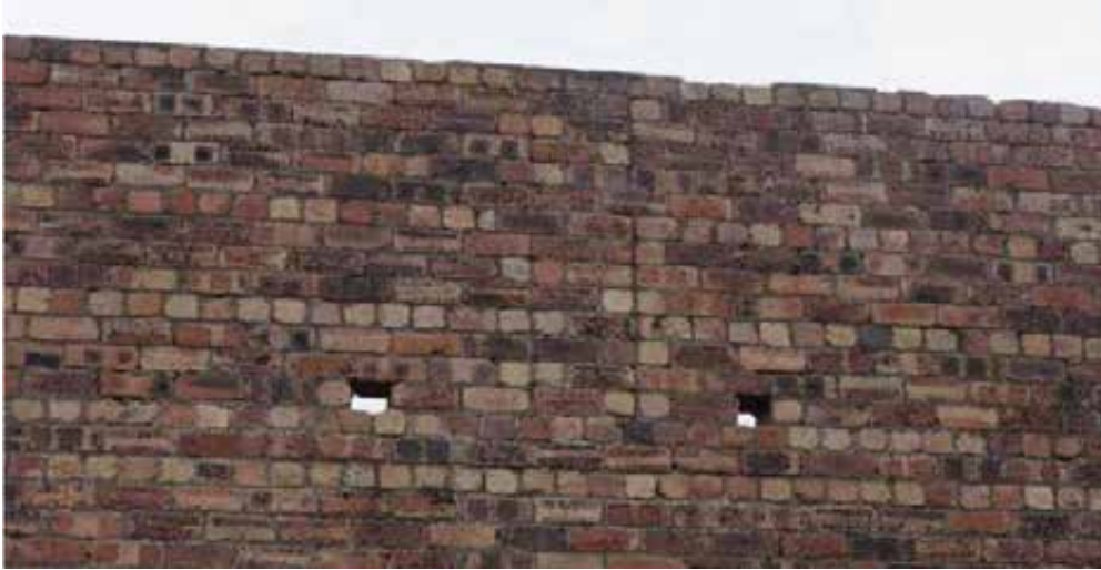
Cracks at higher levels are aligned with the upper piers which are poorly tied to the adjacent thinner single brick thick infilled brickwork.
