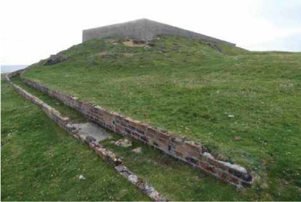
The external brick service trench. Note general deterioration of top courses of its masonry. Note also the loss of material from the embankment about the blast walls.
