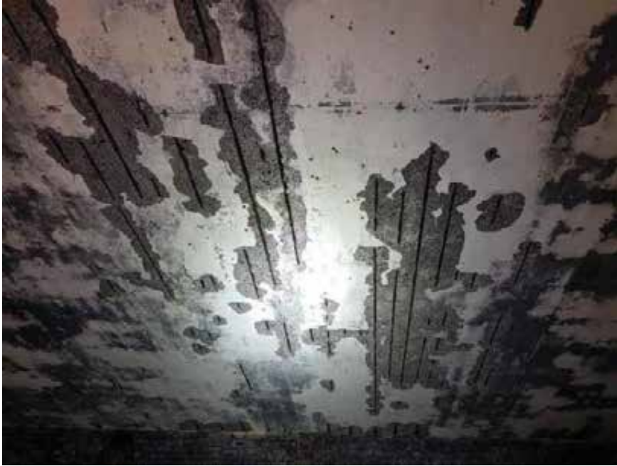
General loss of concrete from the internal soffit of the roof slab.
