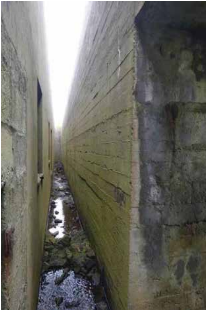
Looking between the blast walls and building proper. Note build up of debris and water.
