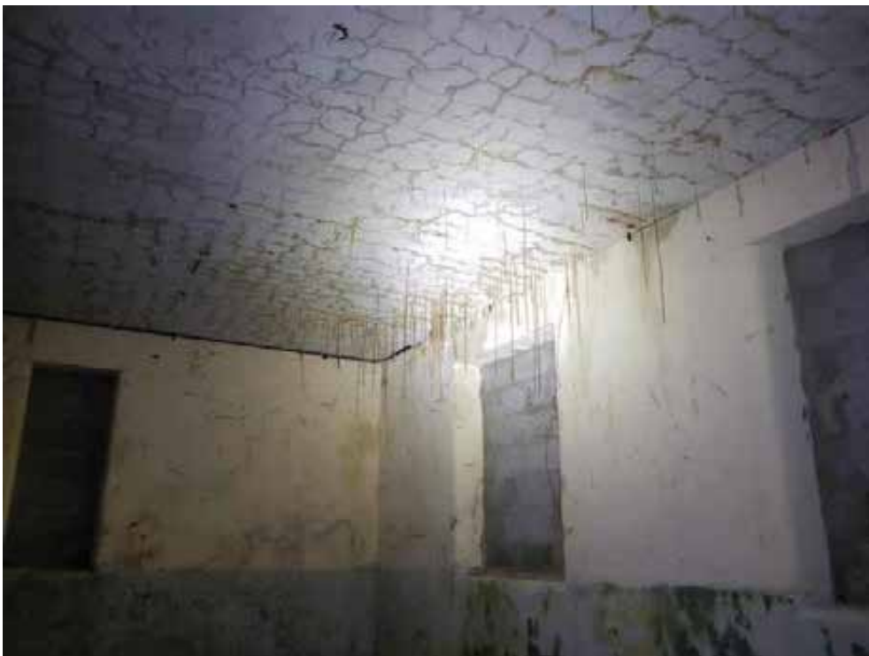
Water ingress through the roof slab obvious, indicated by the stalactites from the roof and cracking of the plaster.
