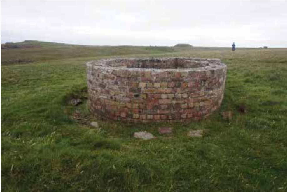
General view from south showing damaged wallhead brickwork and localised failing joints to wall face. Displaced bricks around base of wall.
