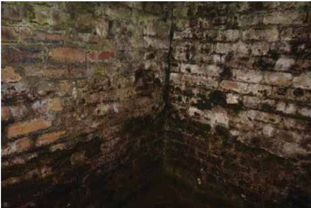
Damp stained brickwork internally from saturated ground conditions.
