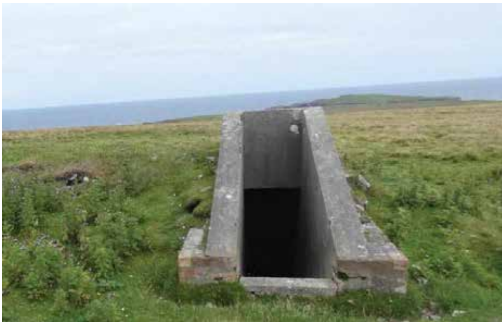
There is only minor damage to the rendered brick tunnel entrance.
