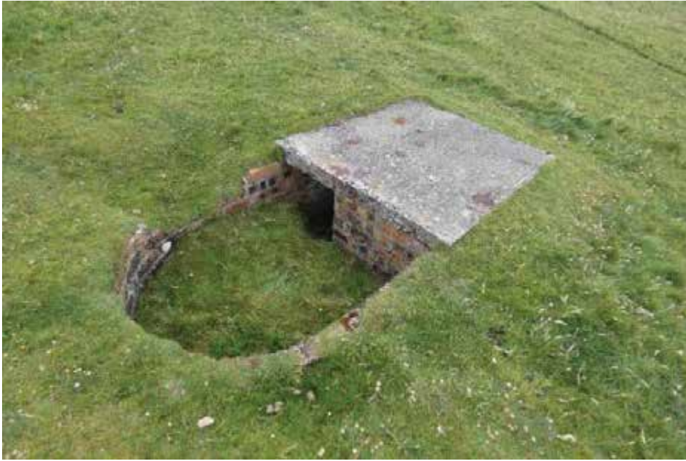
Missing wallhead brick work and defective mortar joints. Minor concrete spalling at slab edge.
