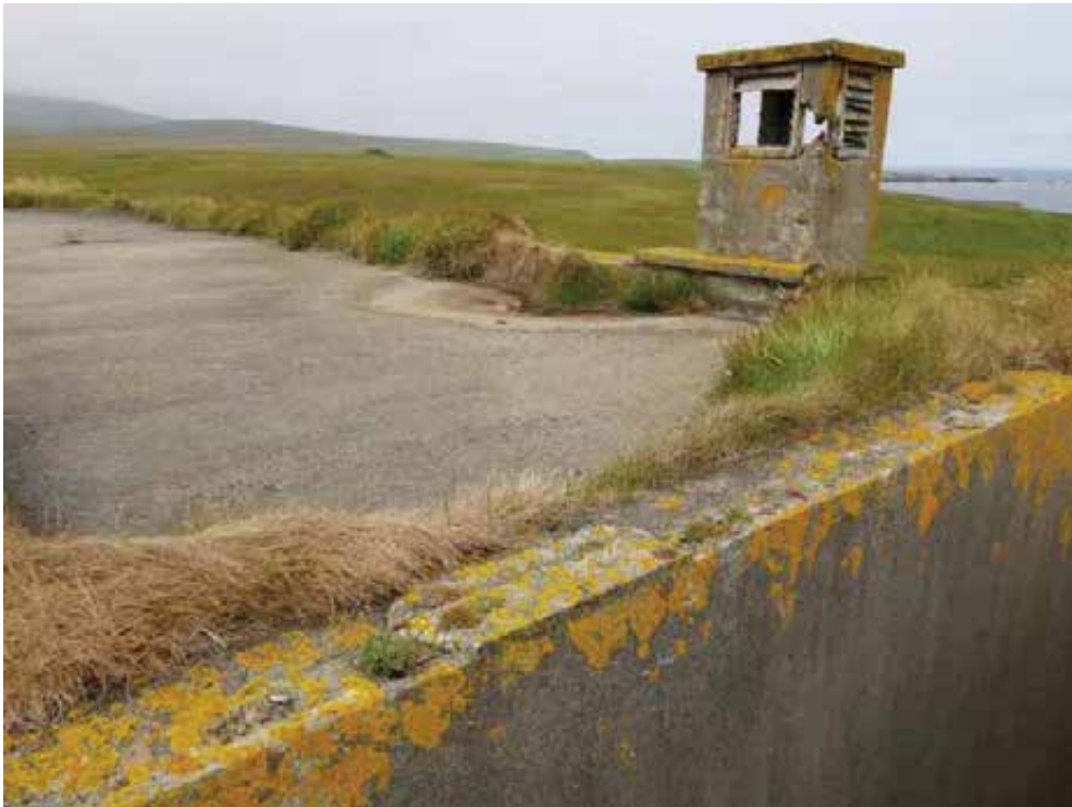
As 6. Note broken leg of RC cap to chimney – see next photo.
