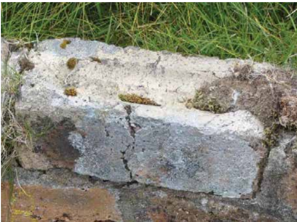
Localised failing joints at curved wallhead.
