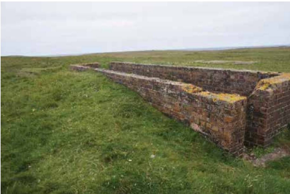
Despite localised failing mortar joints, and damaged and missing brickwork, the structure is in a stable condition.
