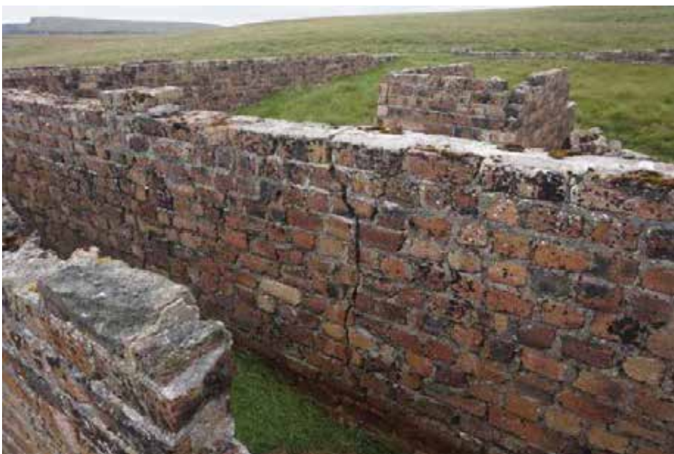
Cracked brickwork to the single brick thick east facing inner skin. Cracks should be repointed to allow future monitoring.
