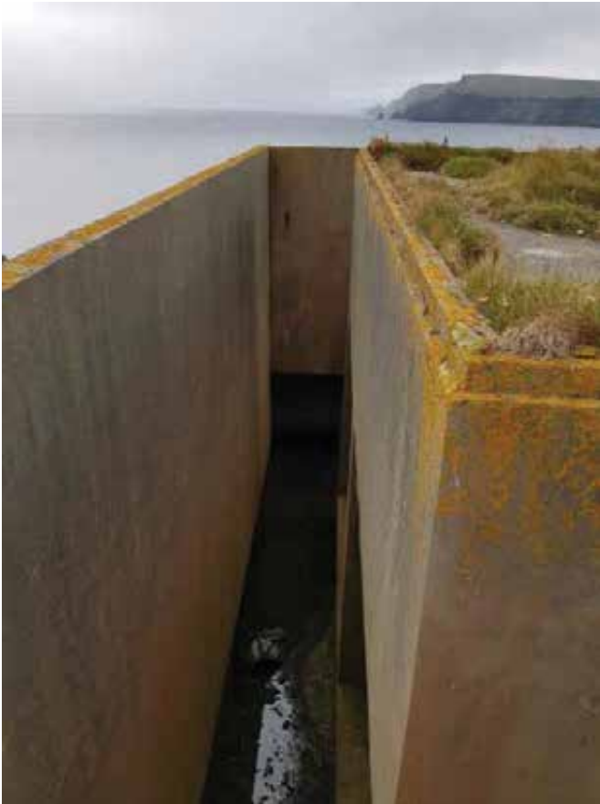
From the top of the embankment looking down into the lightwell between the blast walls and building proper.
