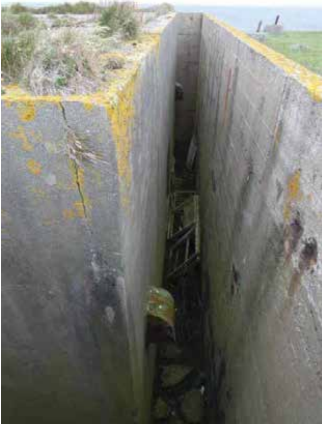
Note the debris across the floor of the perimeter lightwell. Note crack in the render of the building.
