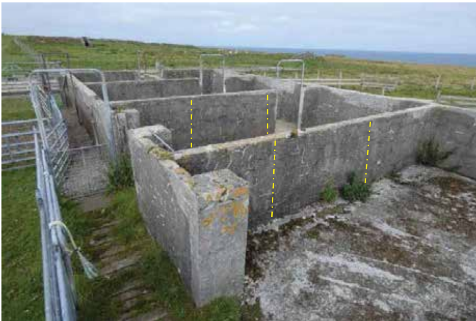
The cement render is extensively cracked and in some areas is supporting vegetation growth. The concrete floor has minor disaggregation and is supporting vegetation growth. The relatively long and slender internal partition walls depend on the integrity of the mortar in their bed joints for their stability. The robustness of these walls can be increased with the introduction of new buttresses at key points (indicated)
