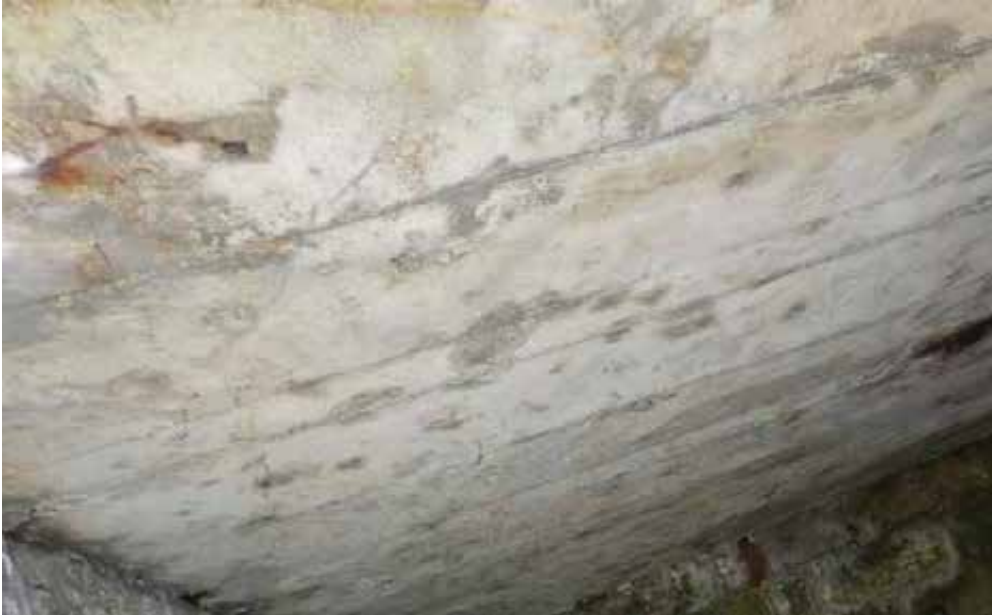
Minor spalling and exposed reinforcement.
