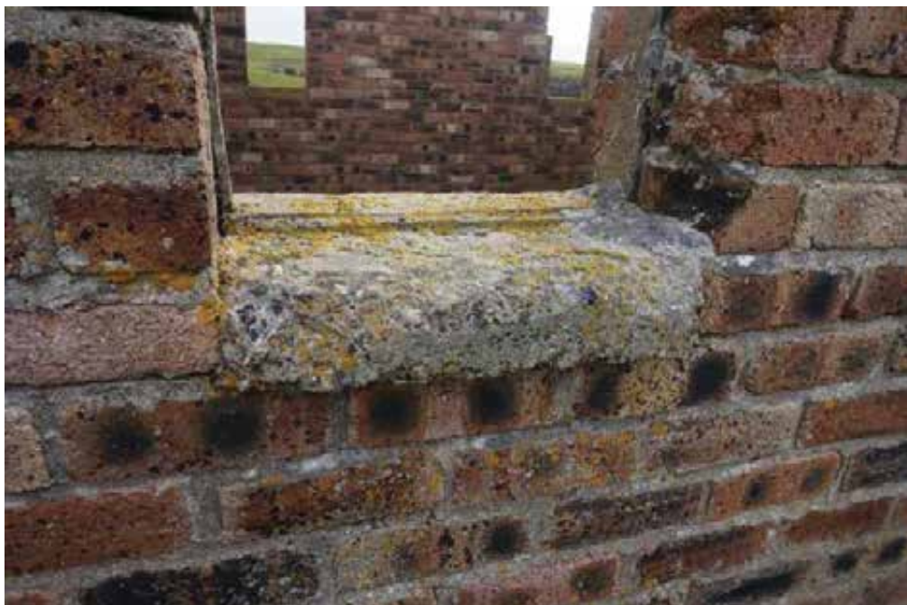
Disaggregating concrete cill.
