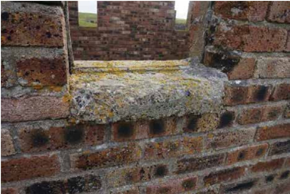
Disaggregating concrete cill.
