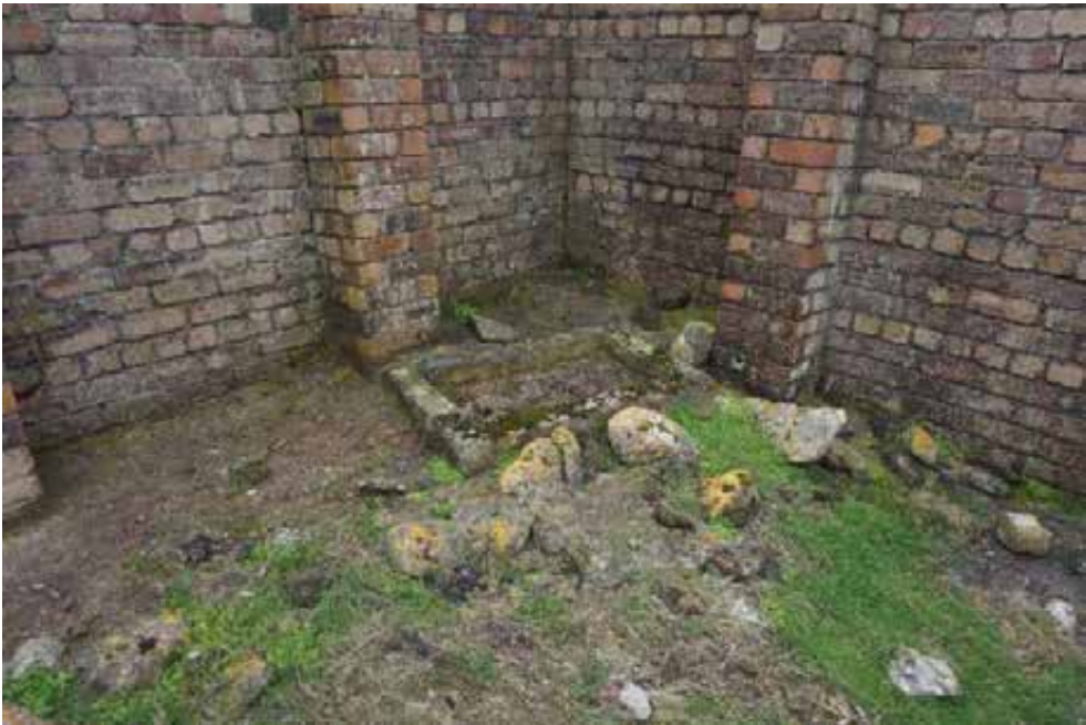
The small rectangle brick structure internally is in good condition. There are loose stones and bricks throughout the grass covered floor internally.
