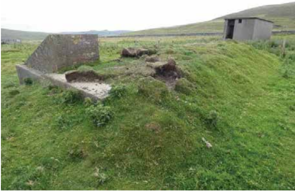
Replacing the missing and damaged earth and turf banking will protect the structure below.
