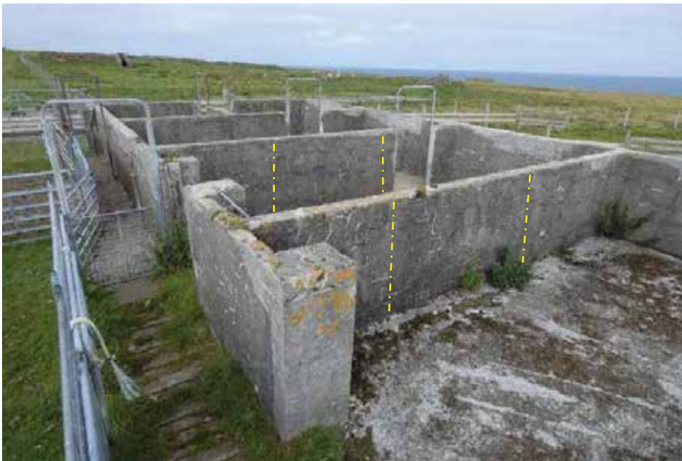
The cement render is extensively cracked and in some areas is supporting vegetation growth. The concrete floor has minor disaggregation and is supporting vegetation growth. The relatively long and slender internal partition walls depend on the integrity of the mortar in their bed joints for their stability. The robustness of these walls can be increased with the introduction of new buttresses at key points (indicated)
