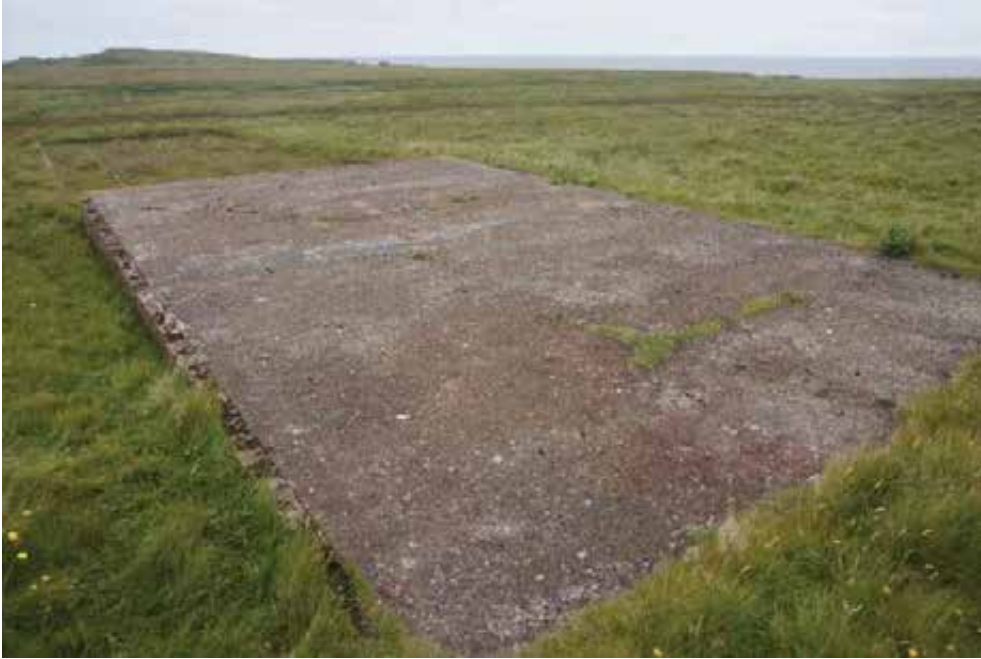
General view from northwest of west portion comprising concrete floor slab surrounded by part buried brick footings.
