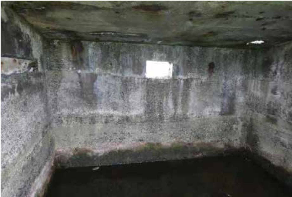
Hairline cracking, rust staining, leaching and discolouration to the walls exacerbated by flooding internally.
