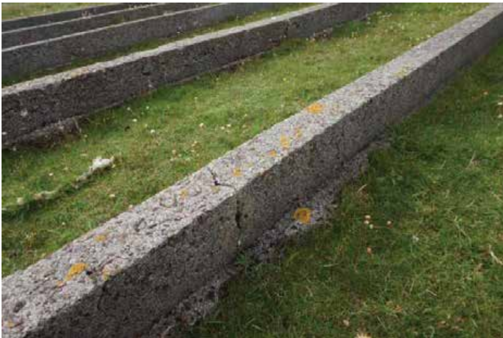
Despite widespread cracking, the walls remain stable.
