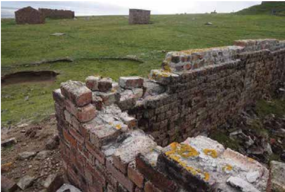
Loose wallhead brickwork and failing joints.
