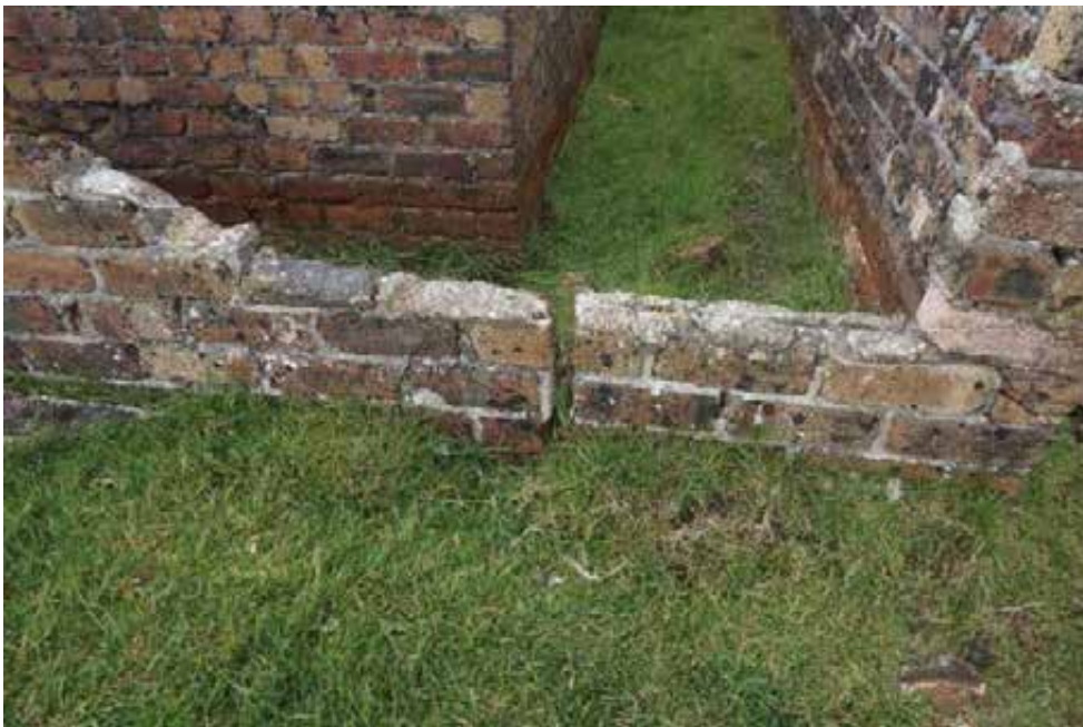
Cracked brickwork to the east facing half brick thick outer skin adjacent to the leaning north wall.
