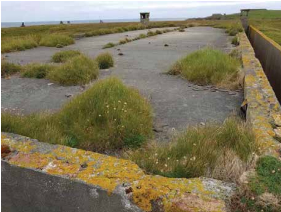
Looking across the roofscape. Note cracked asphalt, vegetation and missing concrete copes from wallheads.
