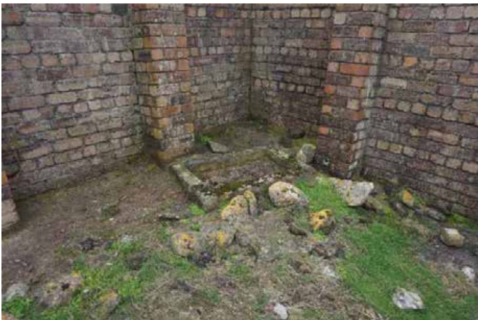
The small rectangle brick structure internally is in good condition. There are loose stones and bricks throughout the grass covered floor internally.
