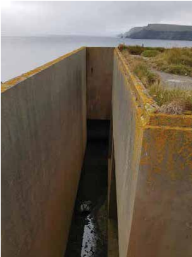
From the top of the embankment looking down into the lightwell between the blast walls and building proper.
