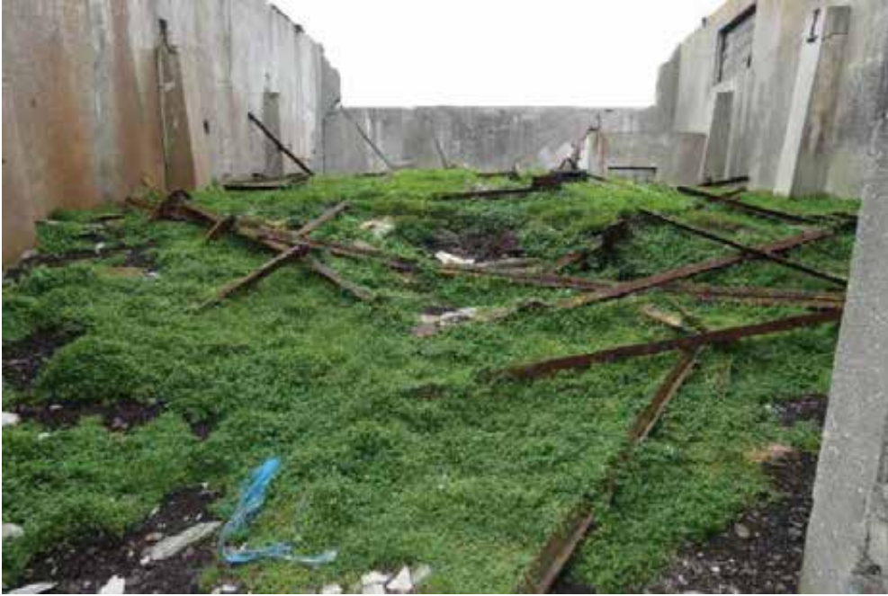
Inside the building. Note remains of the roof structure and asbestos roof tiles.
