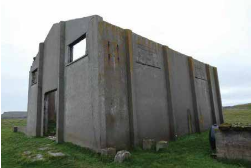
The northeast corner of the building. Note the vertical crack in the east elevation at the corner: there is no continuity between the west or south walls – they are free-standing elements.
