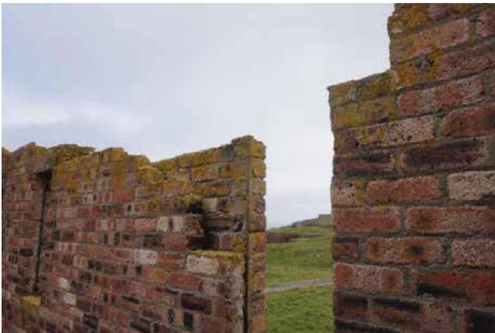
East elevation (internal) with dislodged lintol and fallen wallhead brickwork. To prevent ingress into the cavity, consider resetting the lintol and brickwork to allow the wallhead to be capped in concrete.
