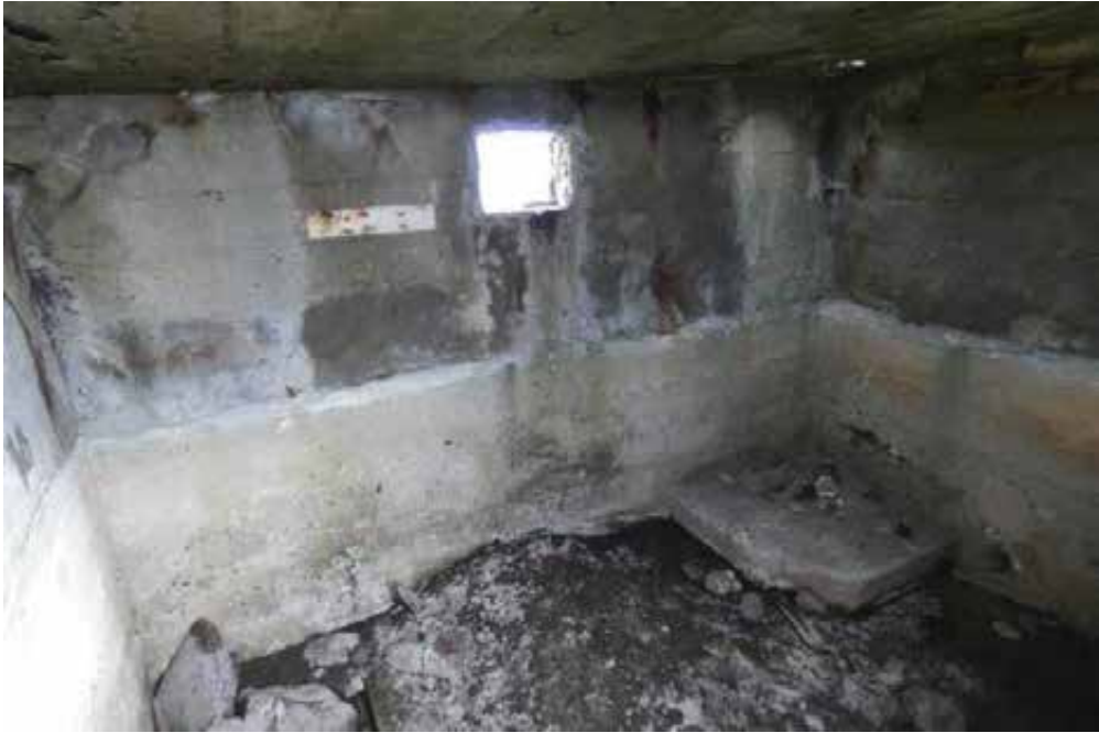
Discoloured and damp stained wall. Floor obscured by accumulated debris.
