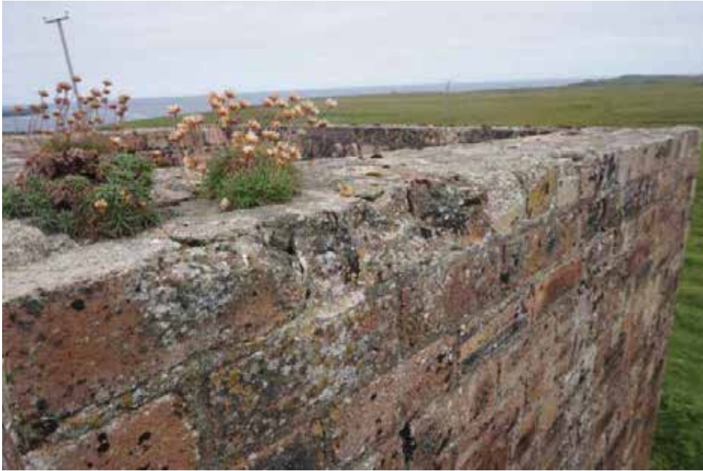
Localised damaged brickwork and defective joints. Vegetation growth at wallhead.
