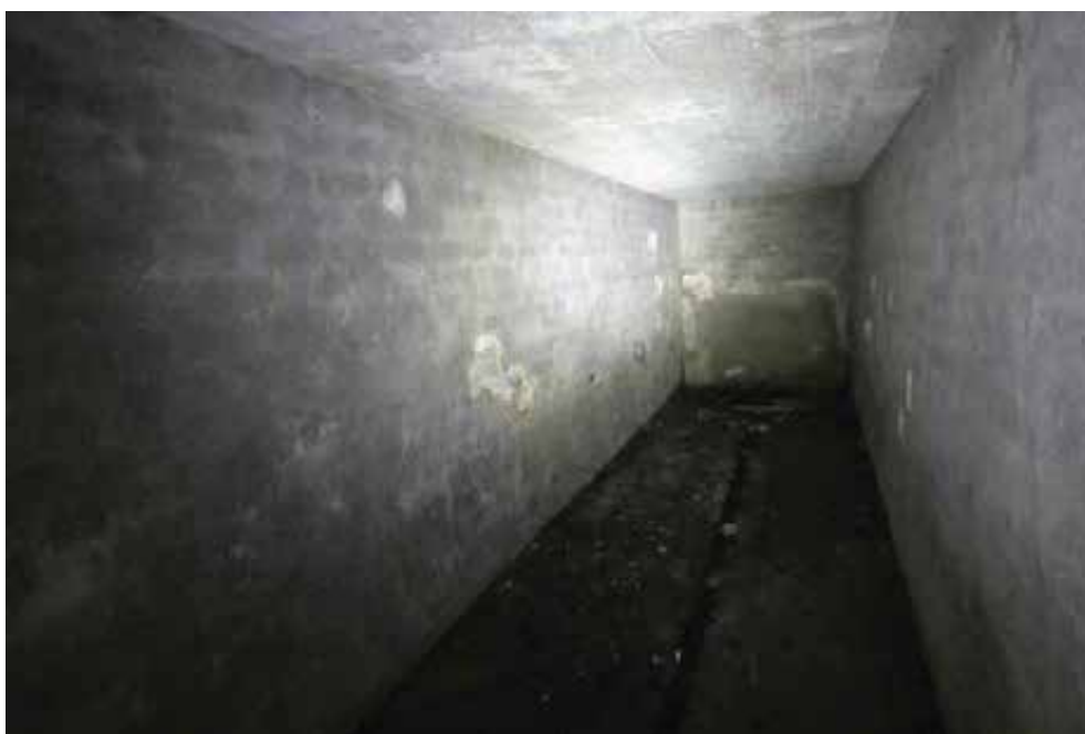
Localised failing render internally.
