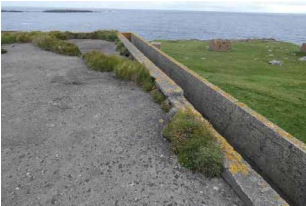
The roofscape. Note missing copes from parapet.
