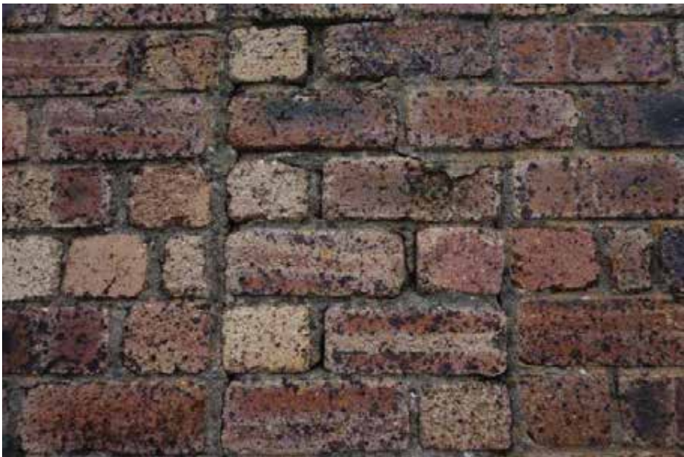
Localised failing wall face joints and minor cracking should be repointed. Note poor continuity between pier (middle of photo) and adjacent panels – see also photos 5 and 6.
