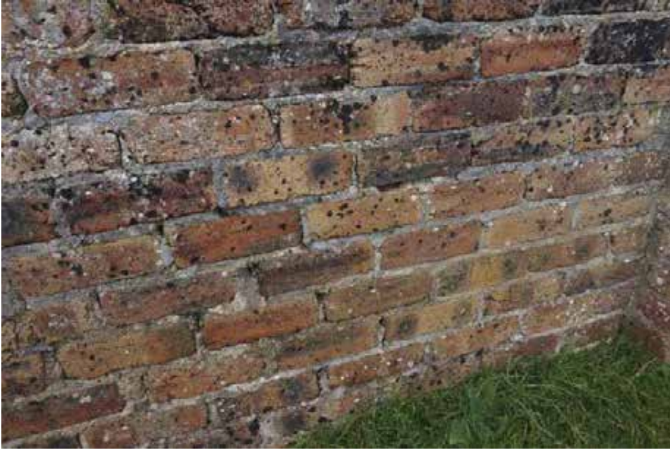
Localised open and failing joints visible on all wall faces.
