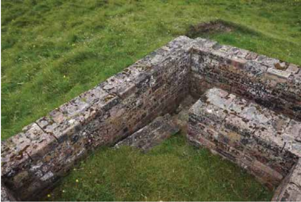
Significant soil and grass accumulations internally and displaced brickwork and concrete.
