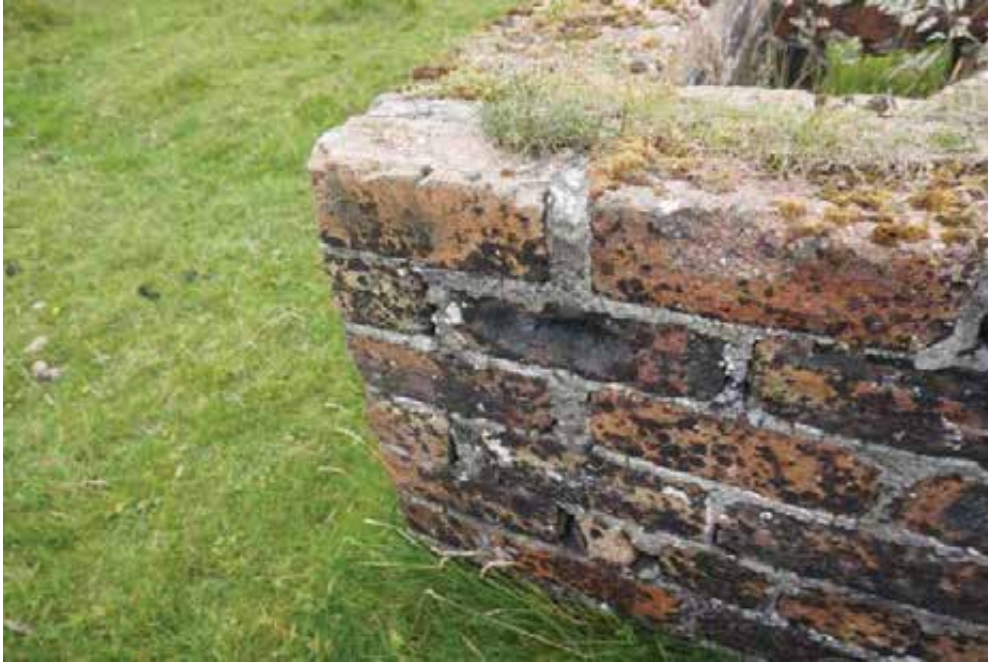
Failing joints to wallhead supporting vegetation growth. Localised damaged bricks and open joints to wall face.
