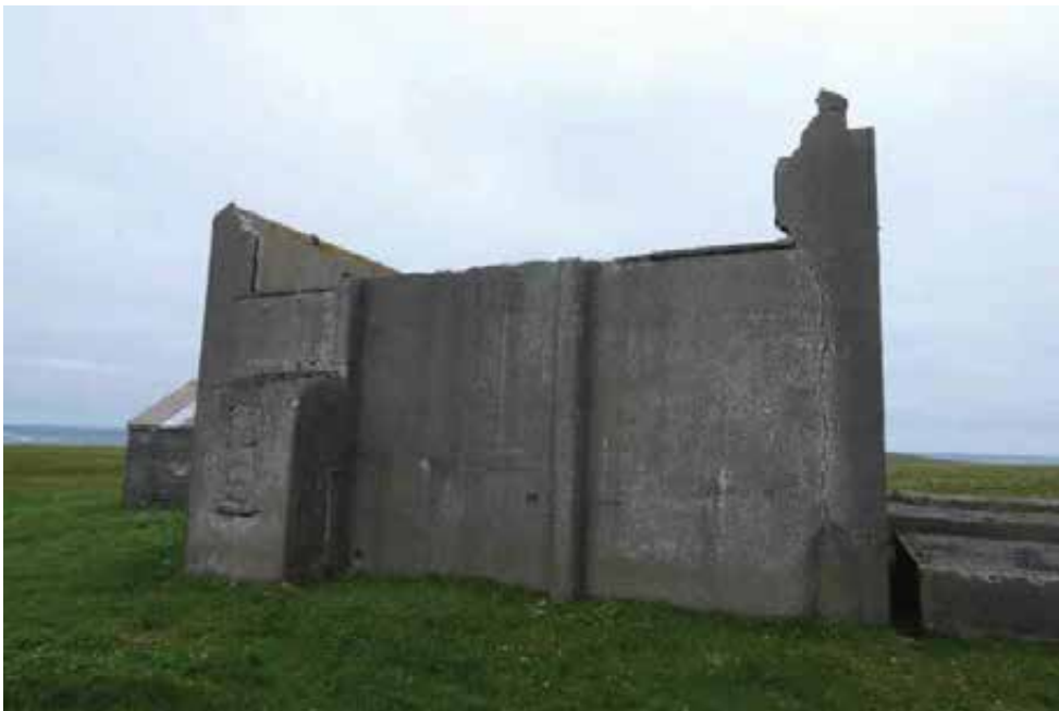
West elevation. The triangular gable has collapsed, falling inwards. Note the full-height crack to the south corner: there is no continuity between the west or south walls – they are free-standing elements.
