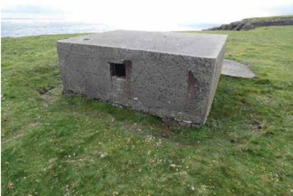
Localised cracking and rust staining.
