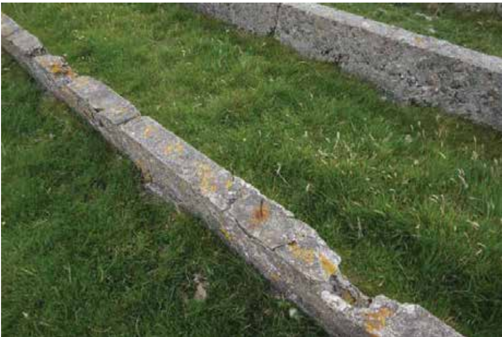
Localised spalling where corroded wallplate fixings survive.
