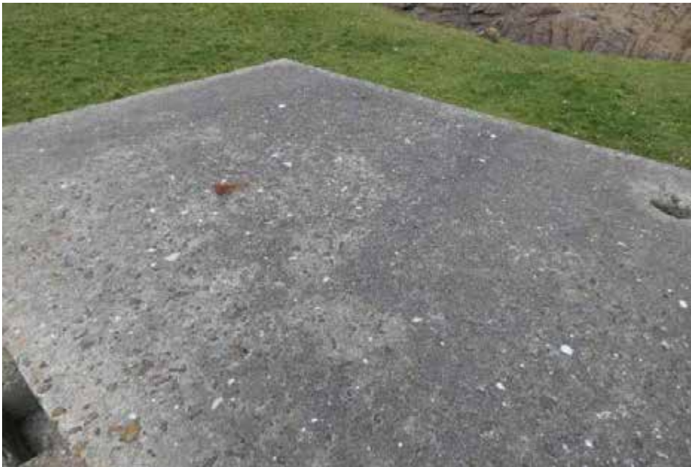
Minor rust staining to the exterior of the roof slab.
