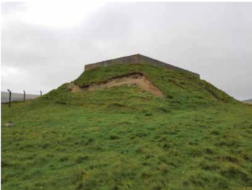
Loss of earth from the embankment owing to burrowing and grazing activities.
