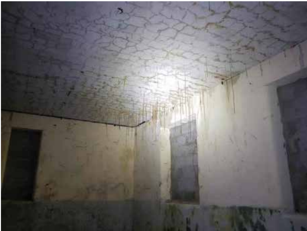
Water ingress through the roof slab obvious, indicated by the stalactites from the roof and cracking of the plaster.
