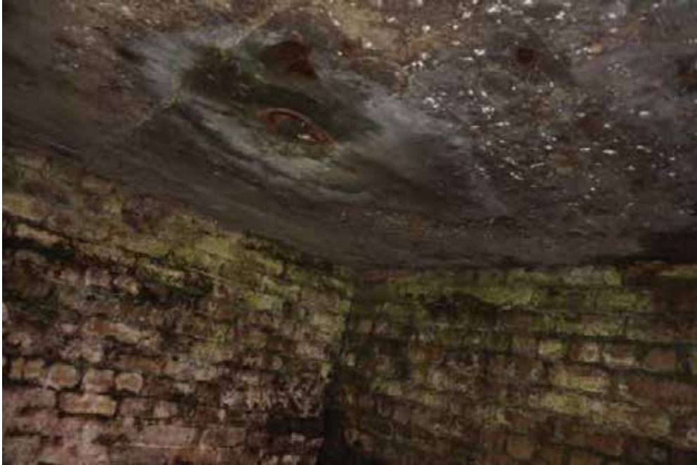
The vent pipe is blocked from above by soil and grass. Localised rust staining was observed on the soffit of the roof slab. No obvious spalling of the concrete.
