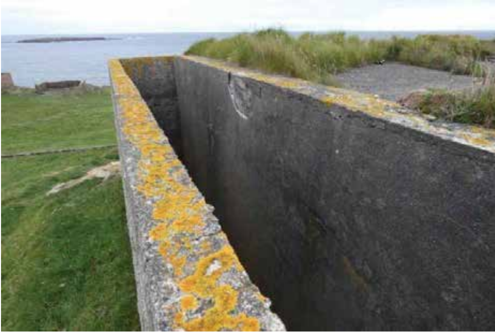
As before. Note the loss of render from the wall of the building.
