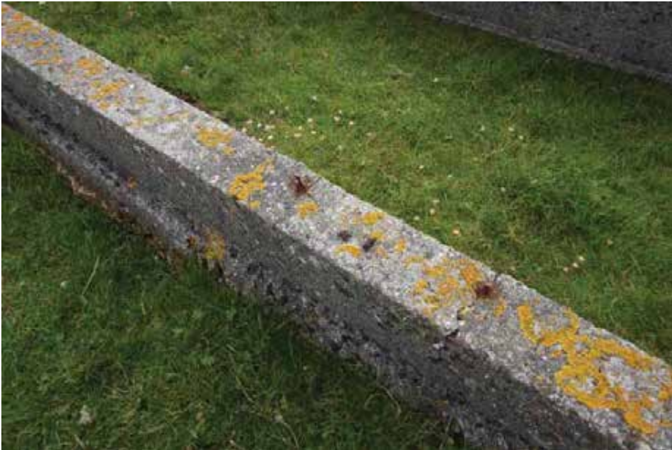
Cracking and spalling in the vicinity of embedded ferrous fixings which would have been used to secure timber wallplates.
