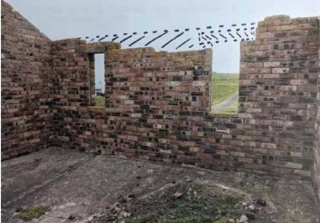
Fig. 12: To minimise water ingress into the cavity wall of the Guard Hut, and the displaced lintel and brickwork could be reinstated to wallhead level to allow capping like that originally placed over the gable wallheads. This work would reduce the rate at which the cavity wall ties will deteriorate.
