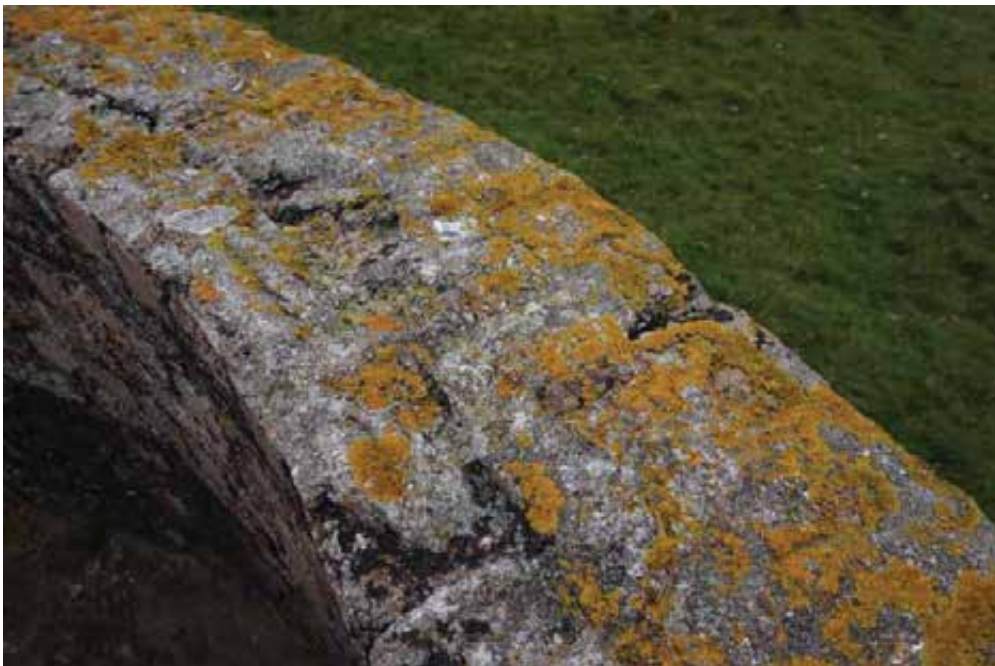
Localised failing skyward facing wallhead joints.
