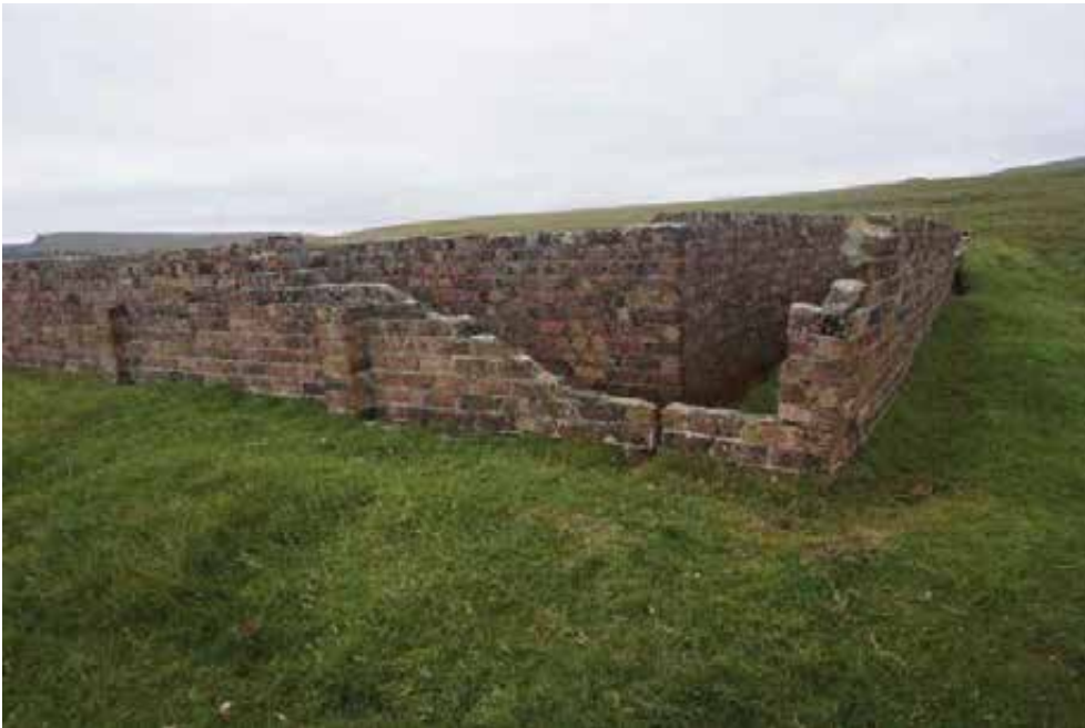
Structural issues in the northeast corner. Vertical cracks on the east elevation of the inner and out skins and a pronounced lean to the north wall of the outer skin. Cracks should be repointed and monitored to assess ongoing movement. The leaning outer skin should either be made safe by extending the earth banking eastwards to prevent further outward rotation or taken down to a safe height. The external wall generally does not have inherent stability generally. This issue should be addressed if increased footfall is expected.
