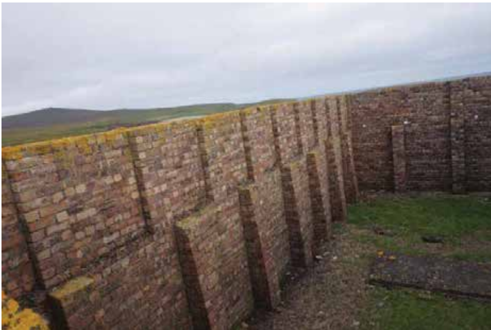
Cracks at higher levels are aligned with the upper piers which are poorly tied to the adjacent thinner single brick thick infilled brickwork. See also Photo 2
