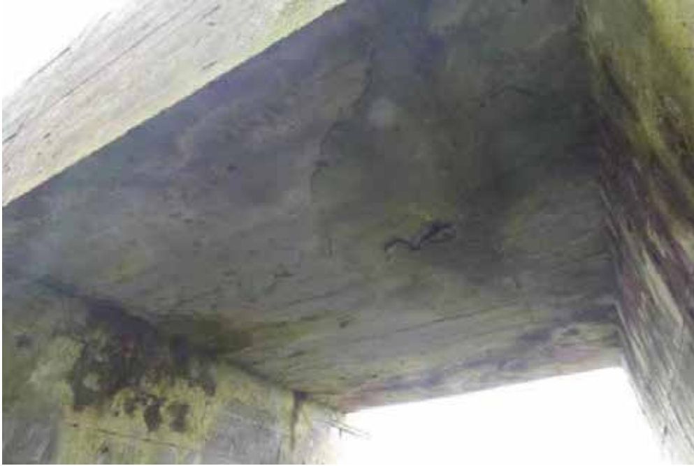
Spalling concrete and render finishes from the soffit of an access tunnel roof.
