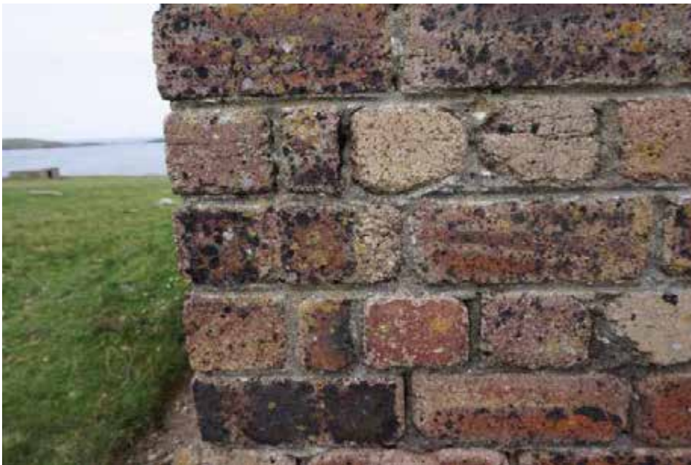
Localised flaking wall face joints and minor cracking should be repointed.
