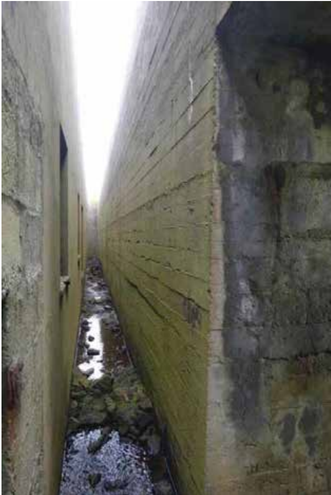
Looking between the blast walls and building proper. Note build up of debris and water.
