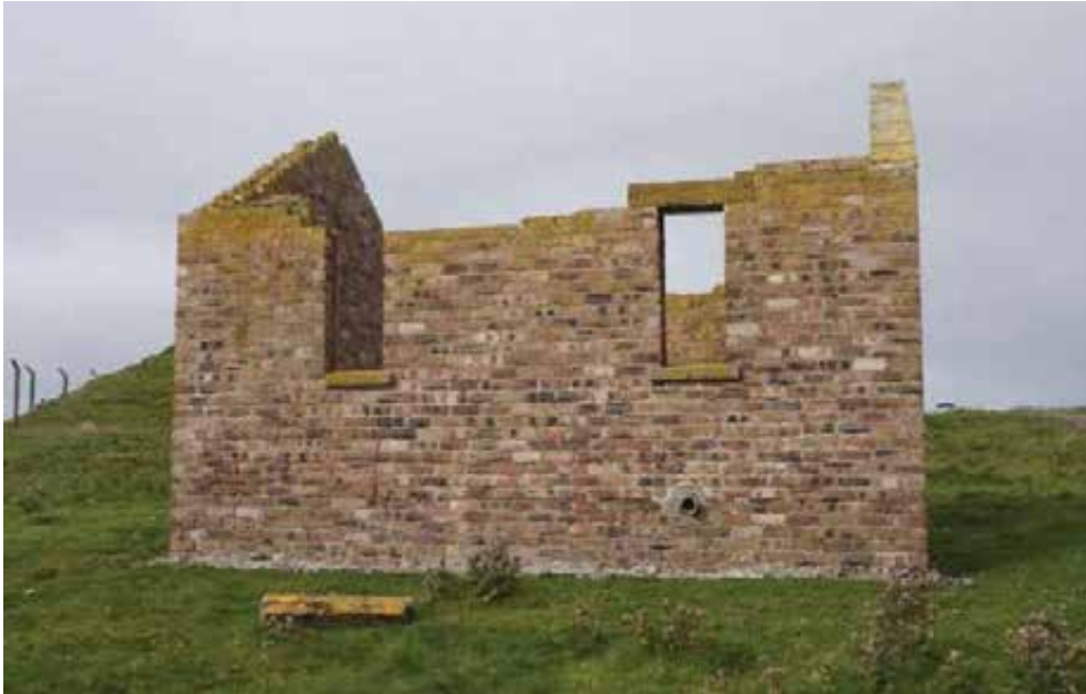
East elevation with dislodged lintol and fallen wallhead brickwork. To prevent ingress into the cavity, consider resetting the lintol and brickwork to allow the wallhead to be capped in concrete.
