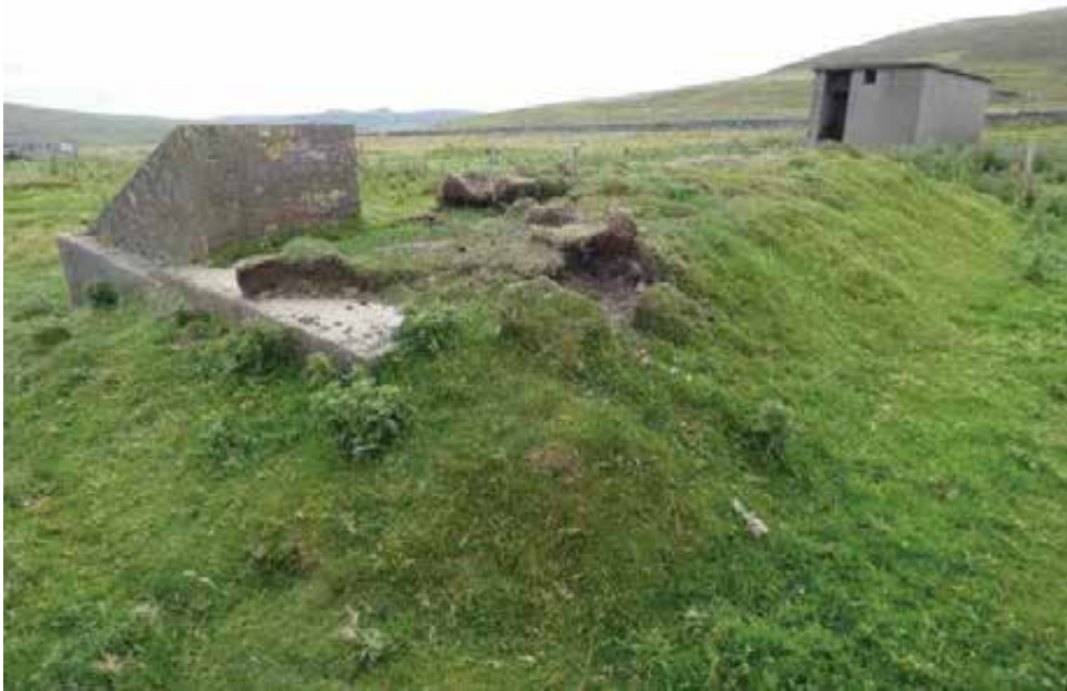
Replacing the missing and damaged earth and turf banking will protect the structure below.
