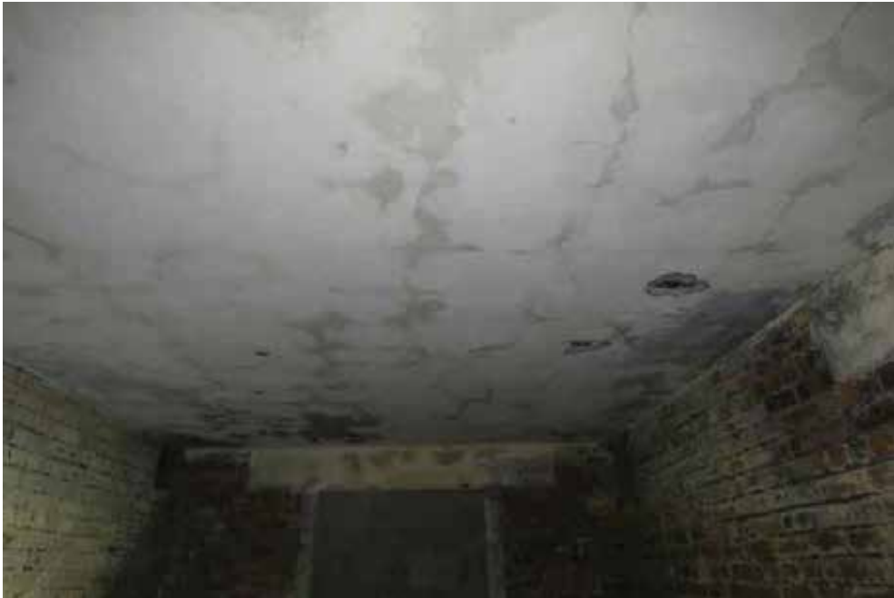
Note cracking of ceiling plaster.
