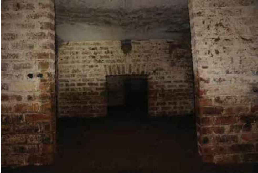
Internal painted surfaces and damp stained and affected by salts from the large accumulations of animal faeces.
