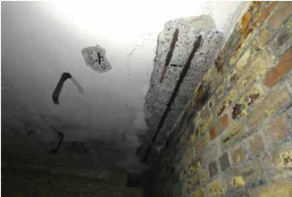
In places, expansive corrosion of reinforcement is causing spalling of concrete from roof soffit.
