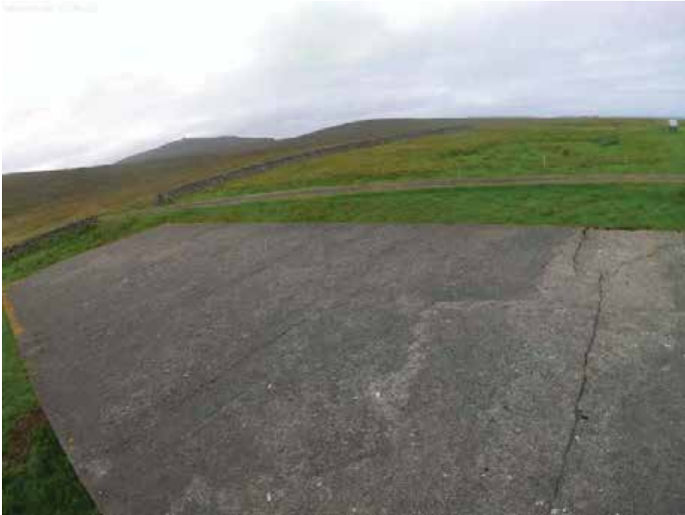
Cracking is visible throughout the exposed concrete roof slab.
