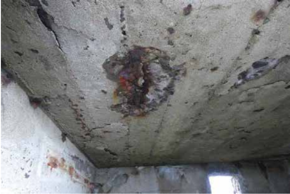
Localised spalling internally exposing corroded reinforcement.
