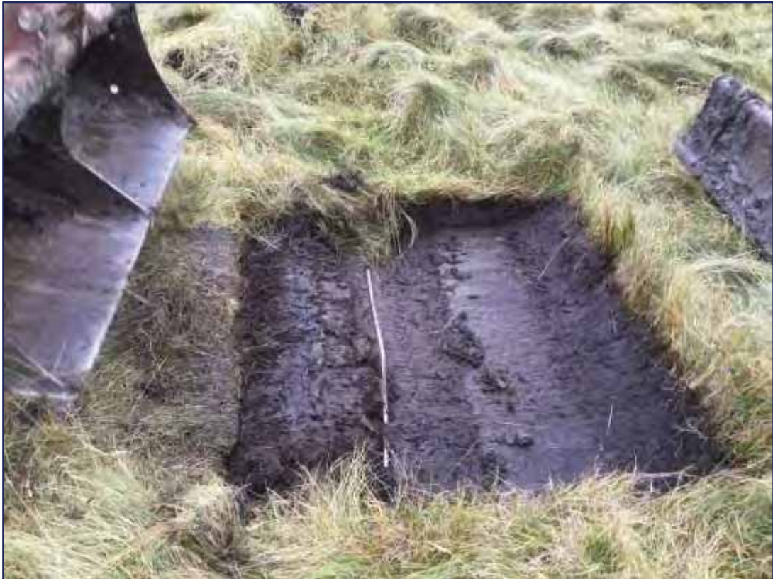
Plate 3: East facing view of TP015 showing the cable found upon opening.
