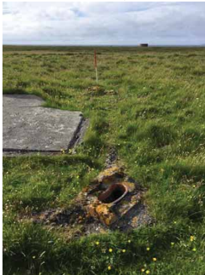
Plate 74: South-east facing view of pipe (Site 427) on the western side of a concrete pad (Site 84b)
