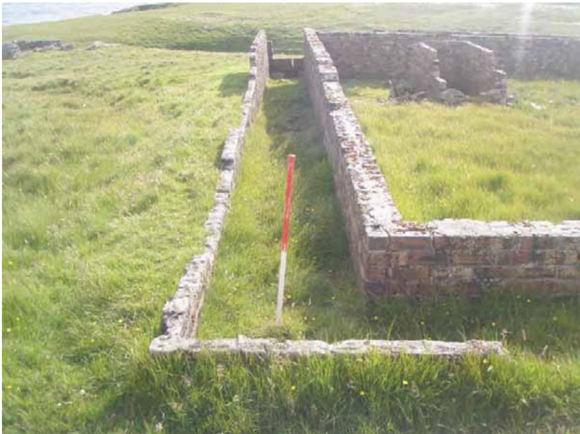
Plate 96: East facing detail of the double brick wall structure (Site 90) showing a crack in the outer, east facing wall
